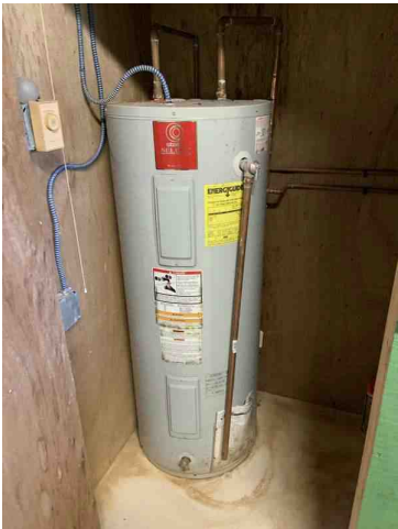
Stable Water Heater
