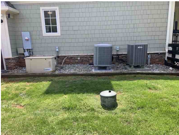
HVAC Units/Buried Propane Tank Access/Standby Generator/Electric Meter
