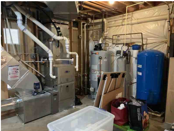
Mechanical and Water Systems
