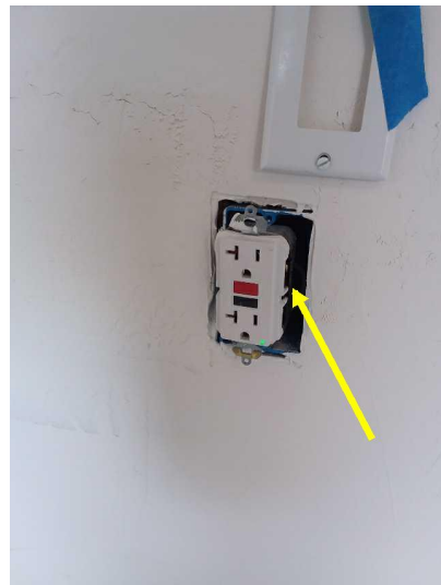
Outlet covers are missing and should be installed.
