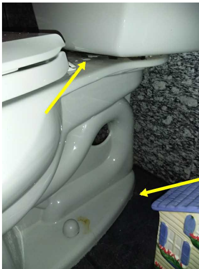
The toilet leaks at the connection between the tank and bowl, which should be repaired.
