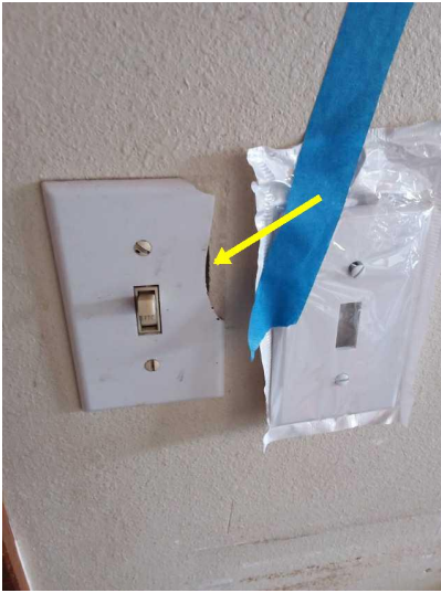
Light switch covers are damaged and should be replaced.
