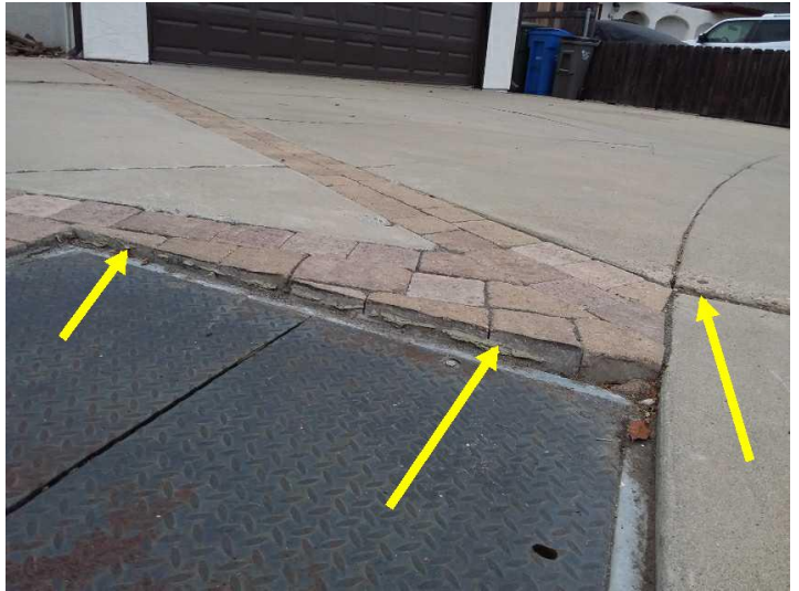
There is one or more offsets in the driveway that could prove to be trip-hazards.
