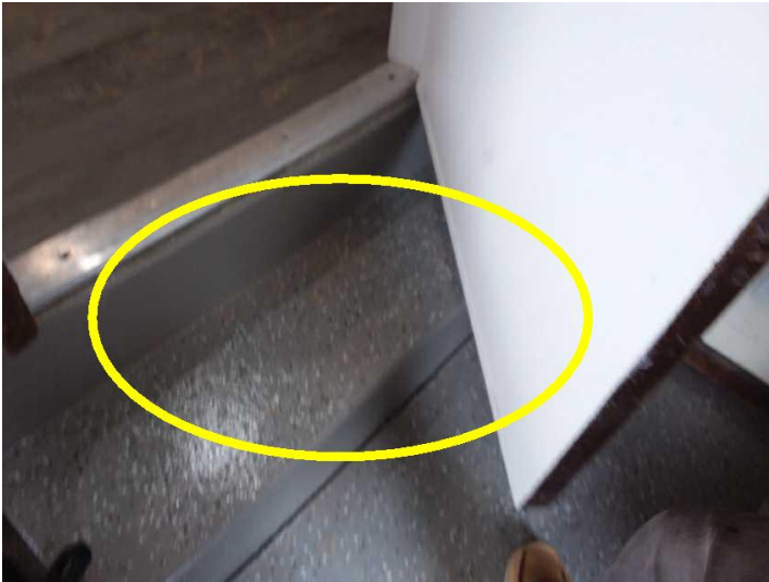
The house entry door opens incorrectly over a step, and should open over a platform the width of the door.
