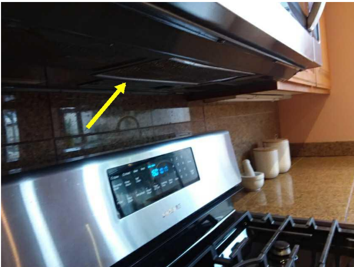
The downdraft exhaust fan light does not respond, and should be serviced.
