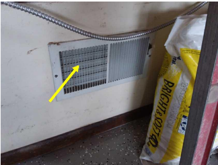
A heat register nullifies the firewall rating and should be repaired.
