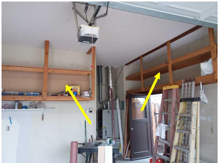
The storage space may have been added without the benefit of a permit, which could stress the roof framing. You may wish to verify this with the sellers. Regardless, you should limit the storage to lightweight items.
