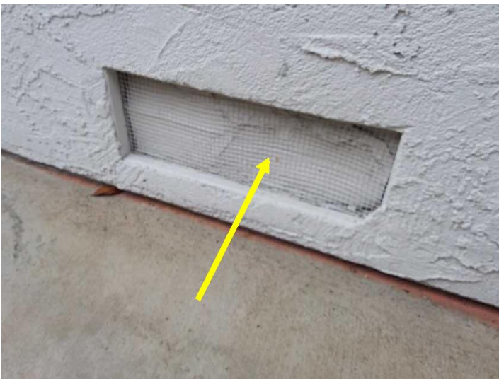
One ventilation port in the wall has been blocked or covered. If they are not uncovered, vehicle engines and combustion appliances could produce noxious by-products, including deadly, carbon monoxide.
