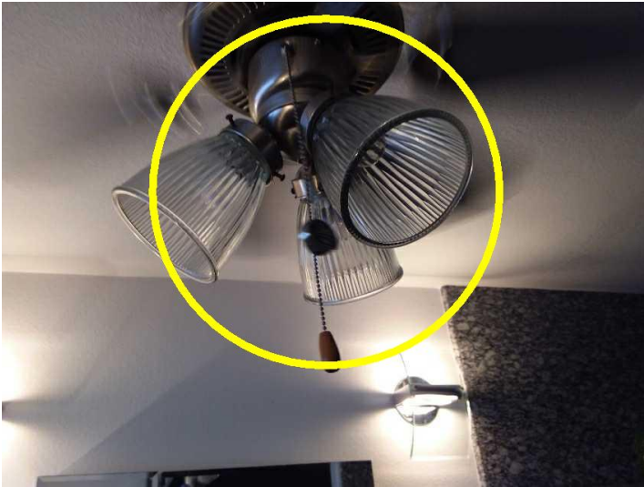
A ceiling light does not respond and should be serviced.
