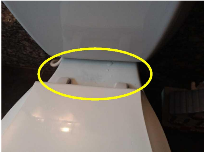
The toilet leaks at the connection between the tank and bowl, which should be repaired.
