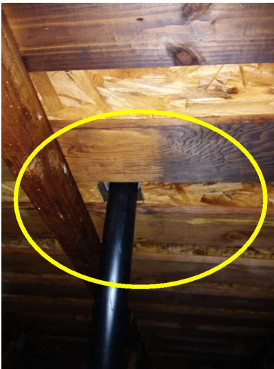
There are moisture stains on the attic ceiling at a roof penetration that indicate a past or present leak. This is a common area for leaks. We are unable to determine if the leak is current, or a past leak, in any case it should be further investigated or explained.
