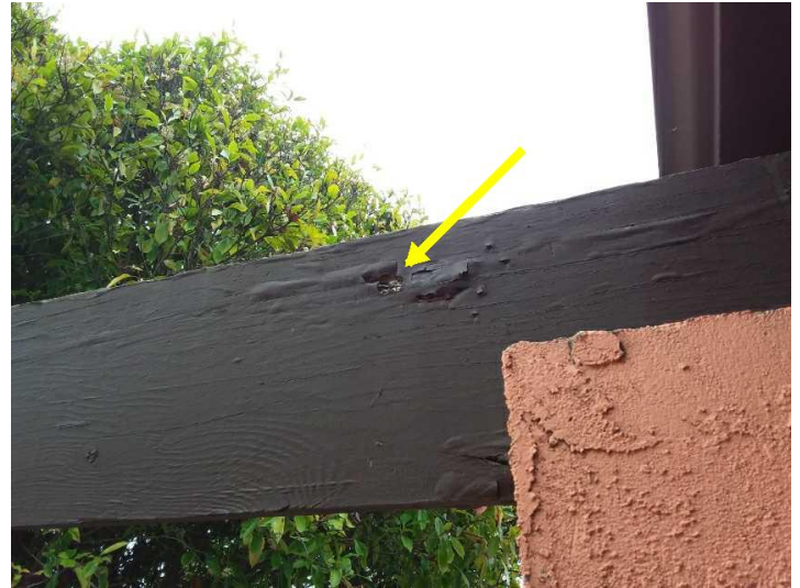
There is damage to the patio cover that should be evaluated by the termite inspector.
