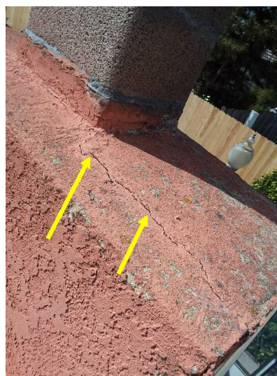
The chimney crown, which is designed to seal the chimney wall and shed rainwater, is cracked and should be sealed.
