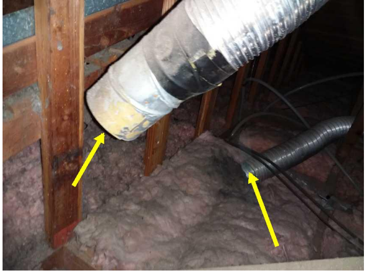
The bathroom exhaust ducts should be extended to an exterior port.
