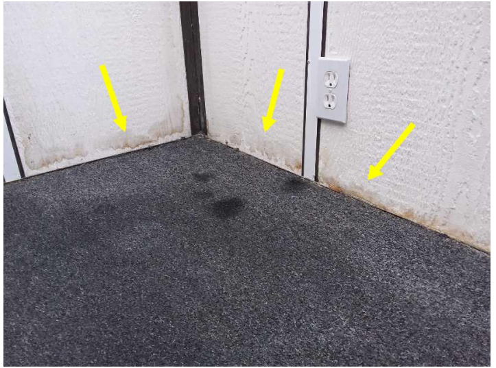
There is a moisture stain on the wall that should be explained or explored further.
