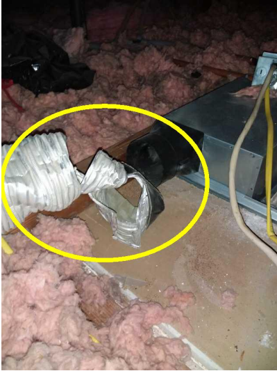
The bathroom exhaust duct is separated, and should be repaired.
