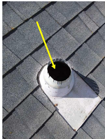
There are penetrations on the roof that are flashed but not sealed. There is a direct link into the attic which should be serviced as a termination cap was removed.
