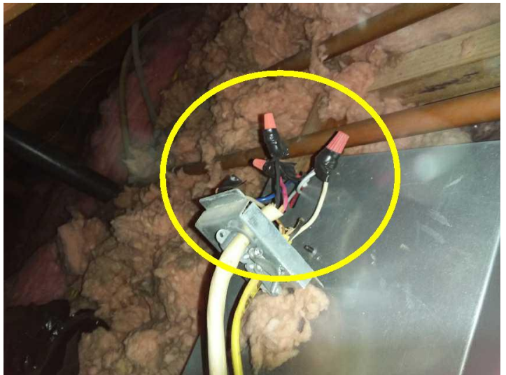
Electrical connections have been incorrectly made outside of junction boxes. All such connections should be made within junction boxes in order to contain any arcing or sparking that could occur, a task that should be completed by a licensed electrician.
