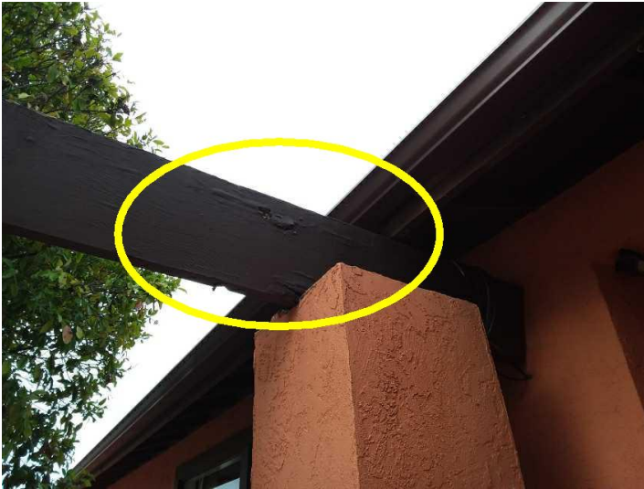
The patio roof-line or beam is deformed and should be evaluated by a licensed specialist such as a framing contractor.
