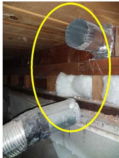
The dryer vent is separated within the foundation crawlspace and should be repaired.
