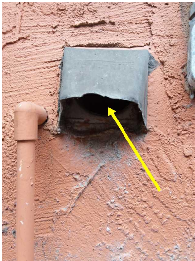
The back-draft on the exterior dryer vent cover is missing, stuck open, or incomplete and should be repaired or replaced.
