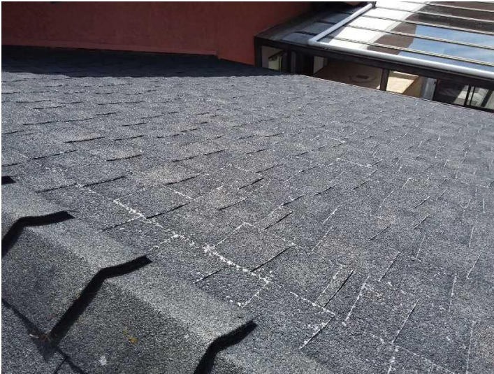
The shingles are losing granules but would not need to be replaced at this time.
