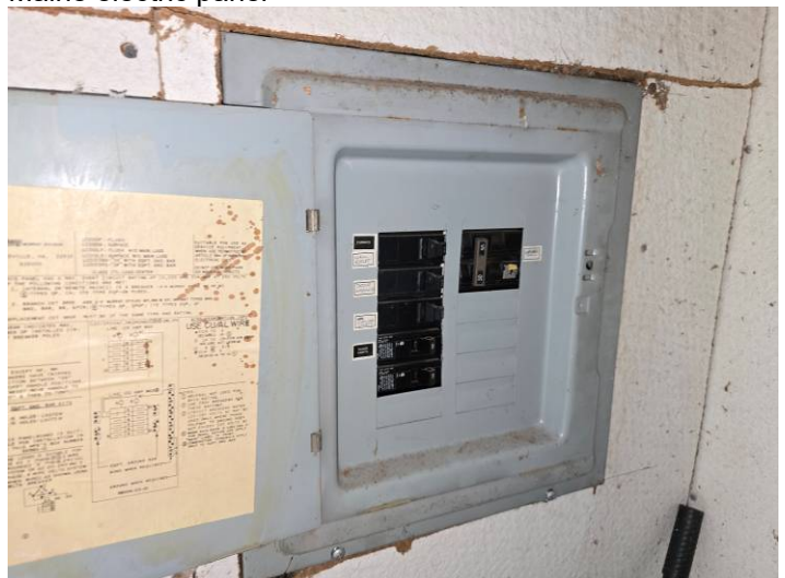
Garage sub panel
