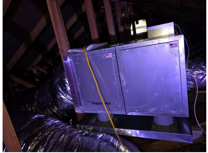
AC unit in the attic space
