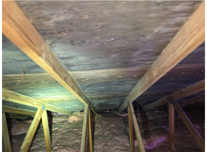
Example of the stained or blackened roof plywood
