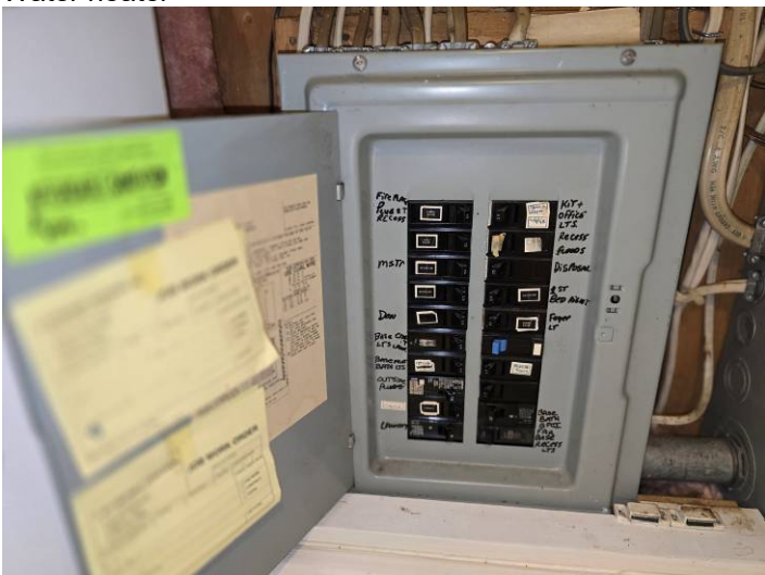
Electric sub panel
