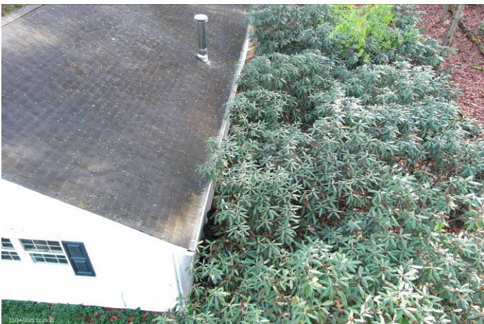
The rear of the garage is overgrown by Rhododendron bushes
