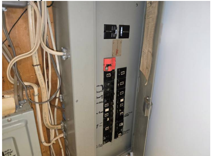
Main electric panel
