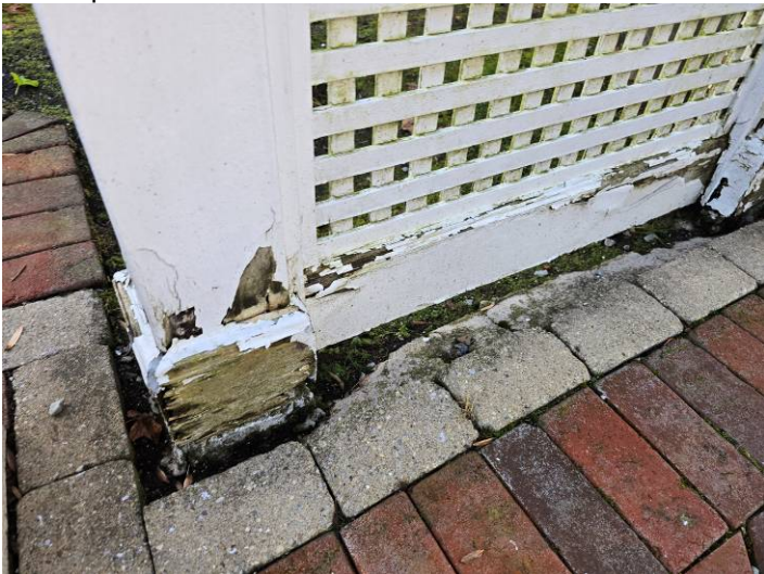
Rotting around the base of the archway to the rear patio
