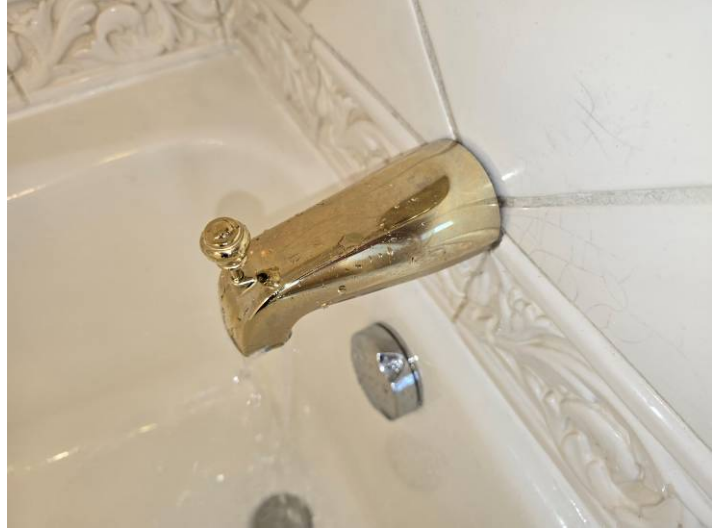
The primary bathtub faucet should be sealed
