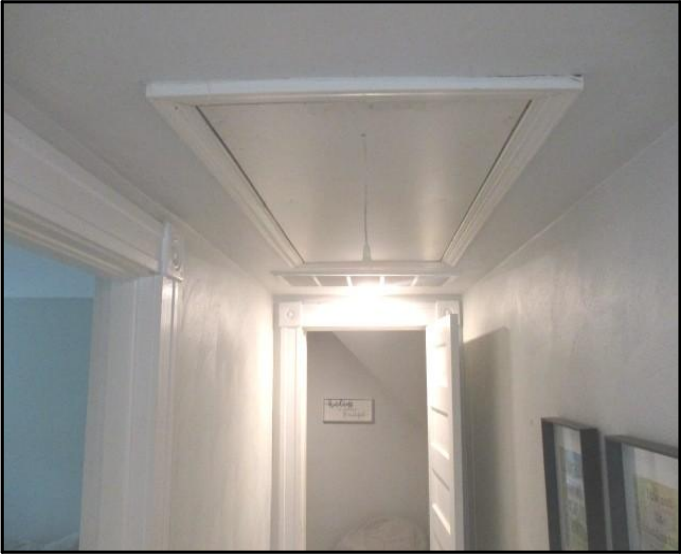
DROP STAIR ATTIC ACCESS
