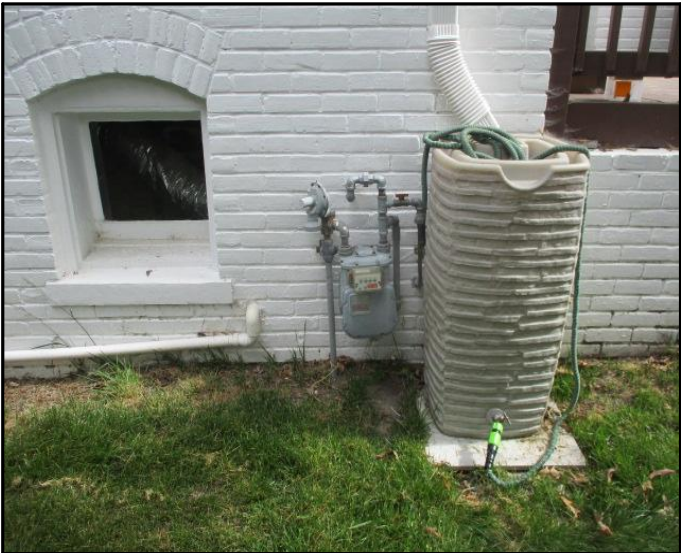
NATURAL GAS METER
