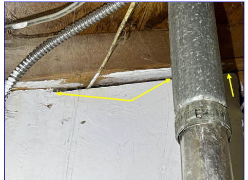
Gap in fire separation wall
