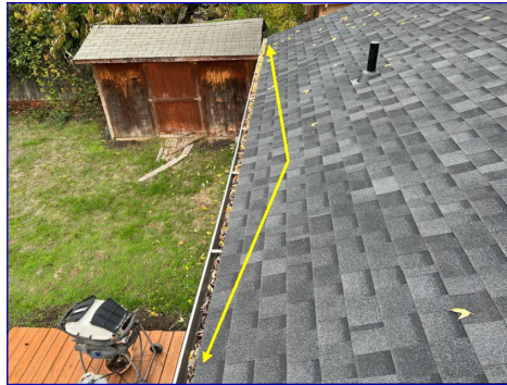
Gutter filled with debris
