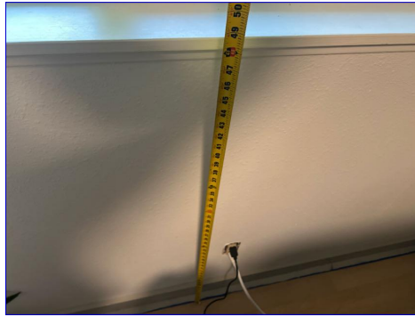
Window sill exceeds 44"
