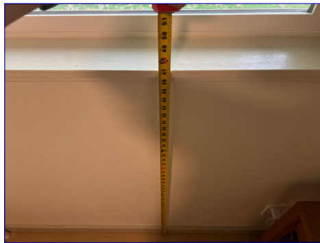
Window sill exceeds 44"
