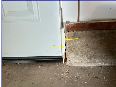
Door does not seal properly
