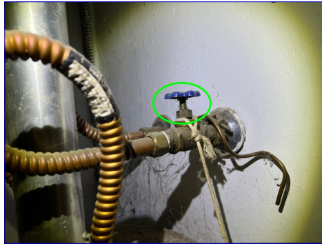
Cold water shut off
