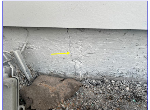
Foundation crack (west)
