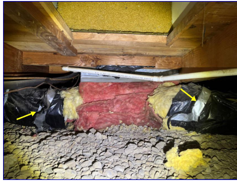
Duct tape on ducting
