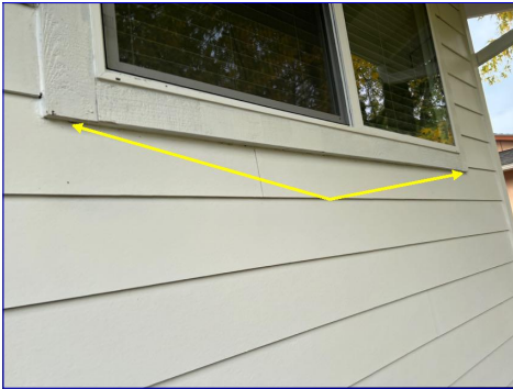
Split caulking at bottom of windowsill
