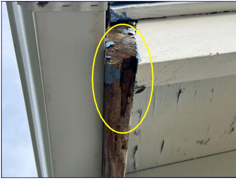
Moisture damage (southwest)
