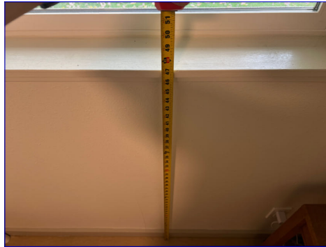
Window sill exceeds 44"
