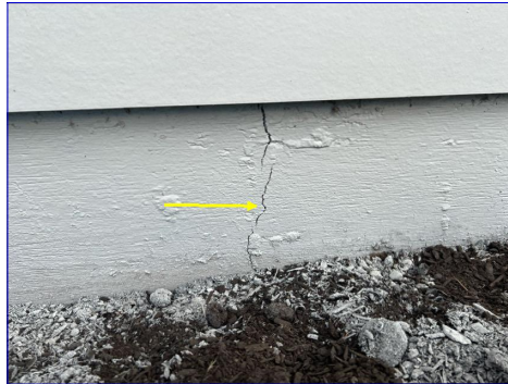
Foundation crack (west)
