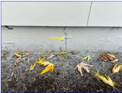
Foundation crack (north)
