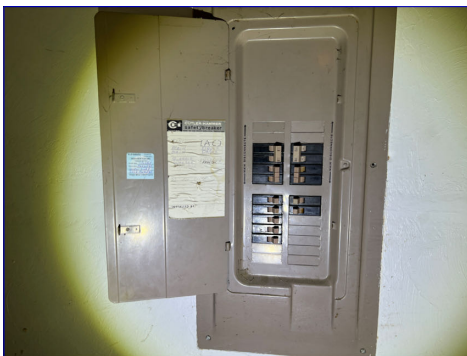
Main electrical panel
