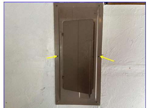
Missing panel screws
