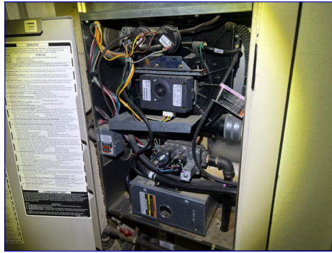
HVAC unit interior
