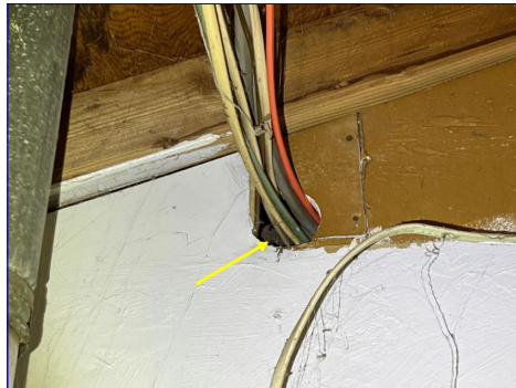
Hole in fire separation wall
