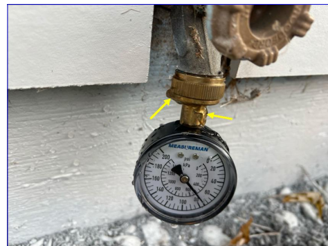
Exterior faucet leaks when connected
