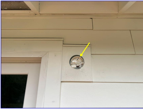
Missing light fixture
