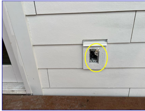
Missing receptacle and weatherproof covering
