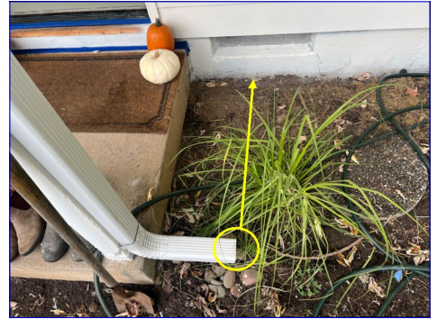
Downspout discharges within 6' of foundation
