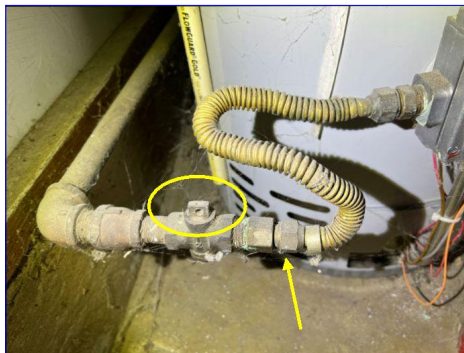
Missing sediment trap
