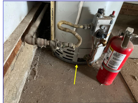
Water heater is less than 18" of floor
