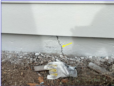
Foundation crack (south)
