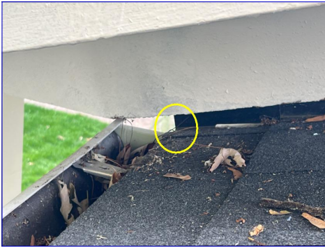
Missing diverter flashing
