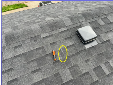
Damage/chipped shingle area
