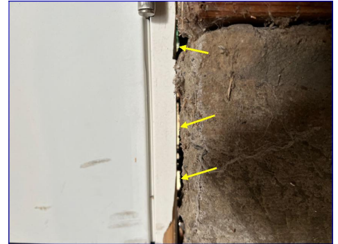
Door does not seal properly
