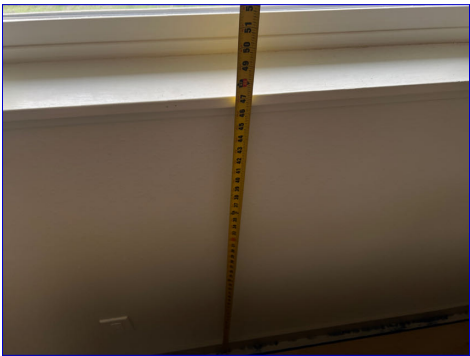
Window sill exceeds 44"
