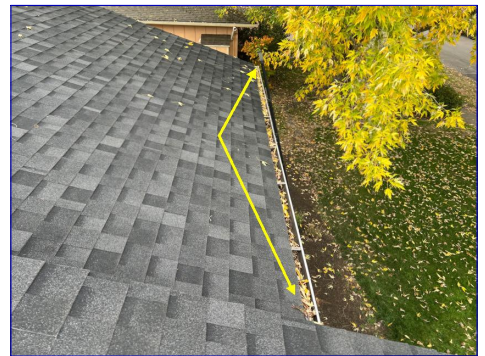
Gutter filled with debris
