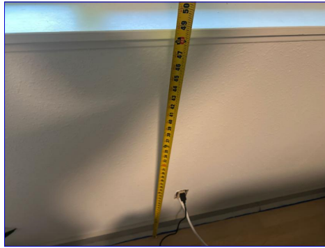
Window sill exceeds 44"
