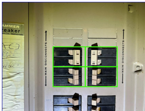
Main electric shut off
