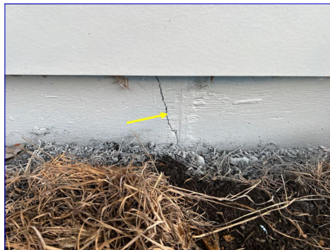
Foundation crack (west)
