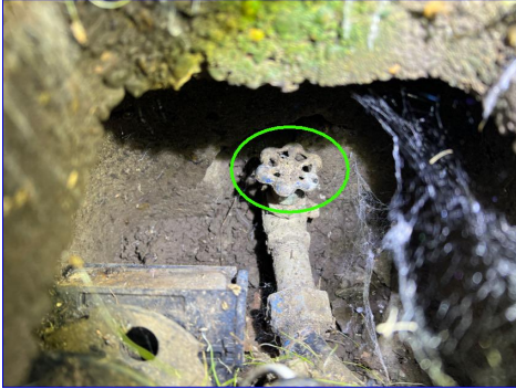
Main water shut off
