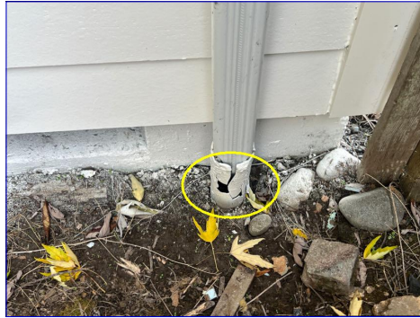
Downspout with damaged leader
