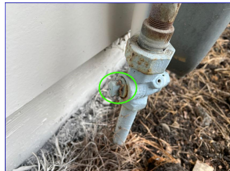
Main fuel shut off
