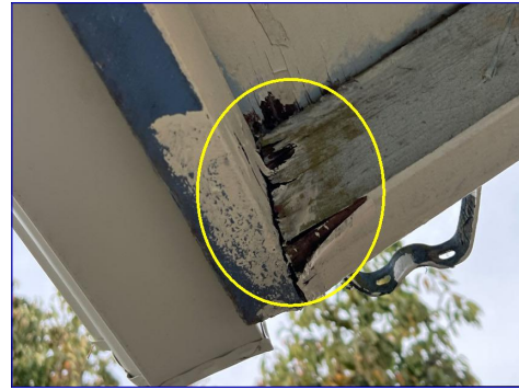
Moisture damage (Northwest)
