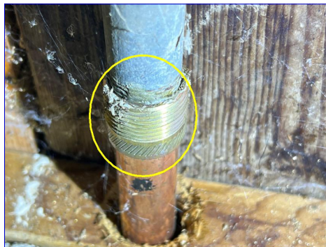
Incorrect metal to metal connection
