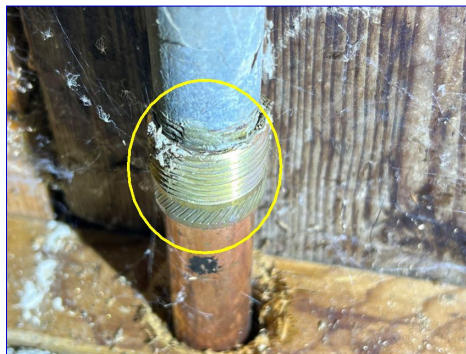
Incorrect metal to metal connection
