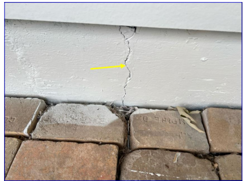
Foundation crack (east)
