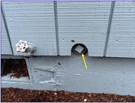
Sewer line clean out
