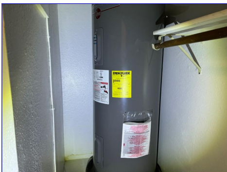
Missing seismic straps
