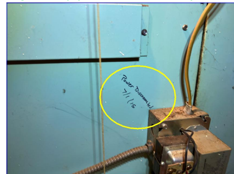
Power was disconnected
