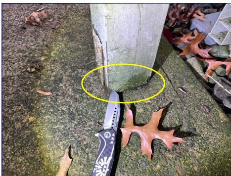
Moisture damage/wood rot
