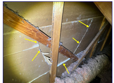
Fire separation between units is compromised
