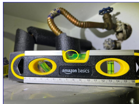
Unit is leaning
