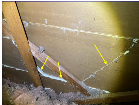
Fire separation between units is compromised
