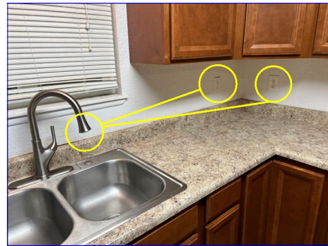
Not GFCI protected (kitchen)
