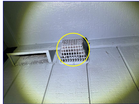
Screen on dryer exhaust vent termination
