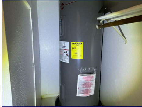
Missing seismic straps
