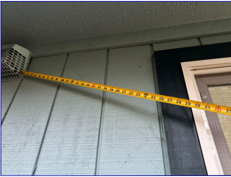
Dryer vent termination too close to opening
