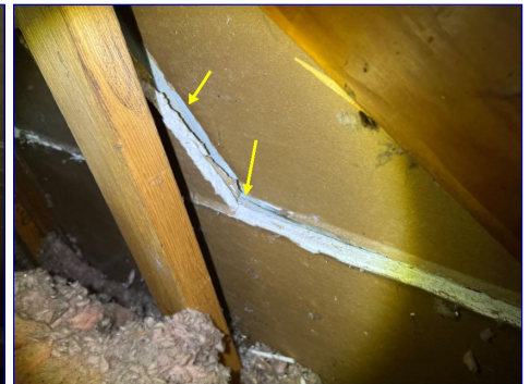
Fire separation between units is compromised
