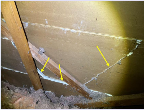
Fire separation between units is compromised
