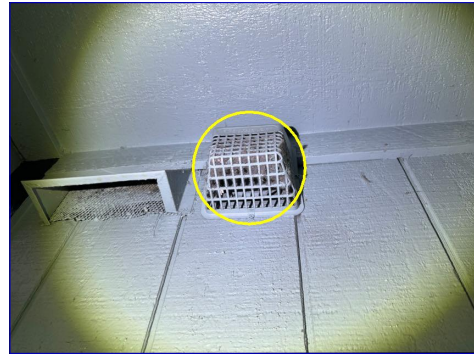
Screen on dryer exhaust vent termination
