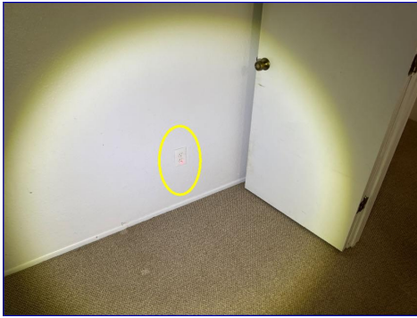
Loose receptacle(s) (Bedroom 1)
