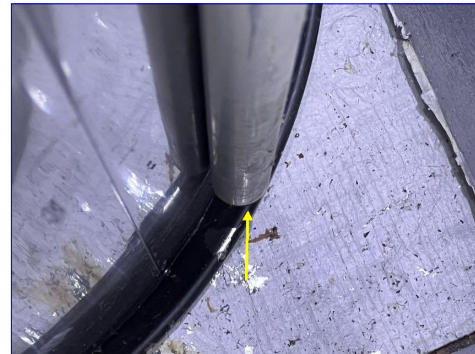
Discharge pipe not aligned with drip pan
