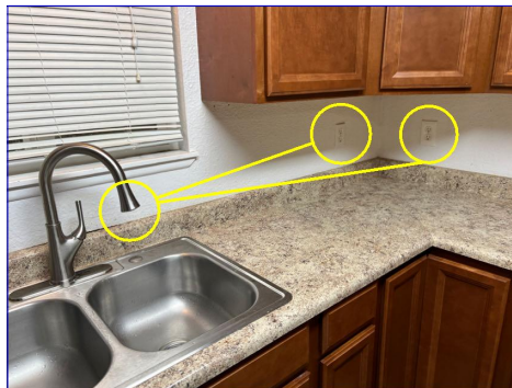
Not GFC protected (kitchen)
