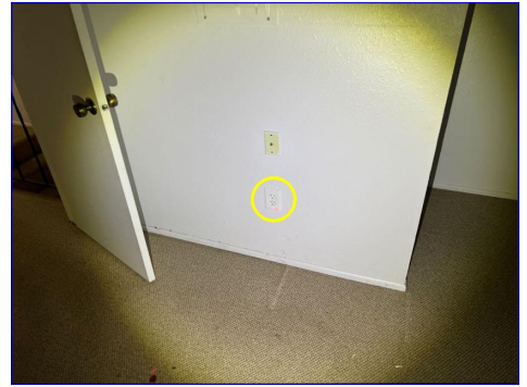
Loose receptacle(s) (Bedroom 2)
