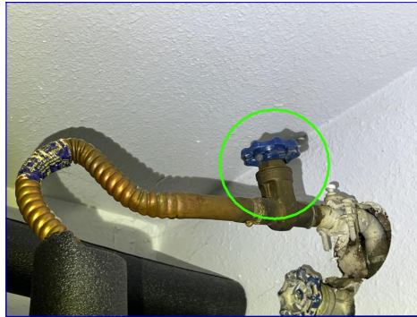
Cold water shut off
