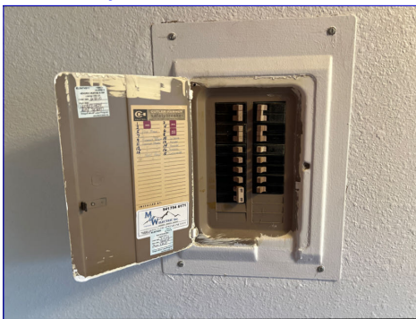
Main electric panel
