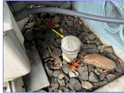
Sewer line clean out
