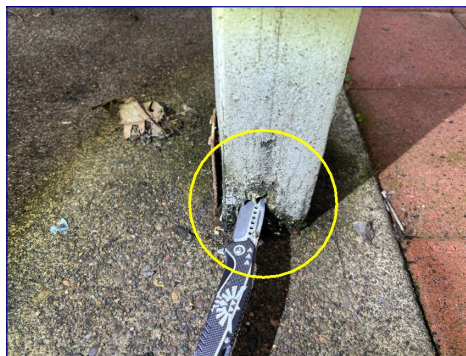
Moisture damage/wood rot
