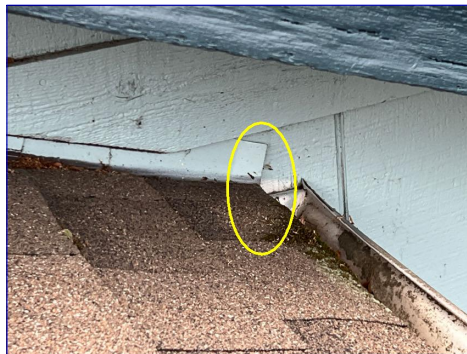
Undersized diverter flashing
