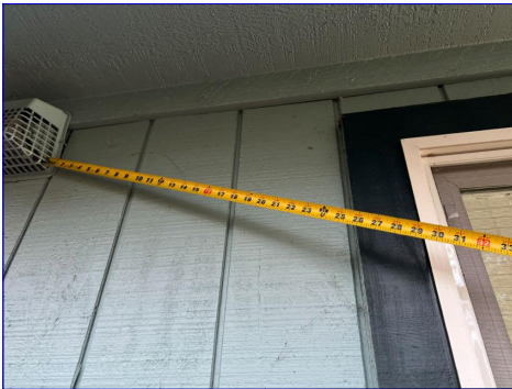
Dryer vent termination too close to opening
