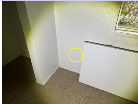
Loose receptacle(s) (Bedroom 2)
