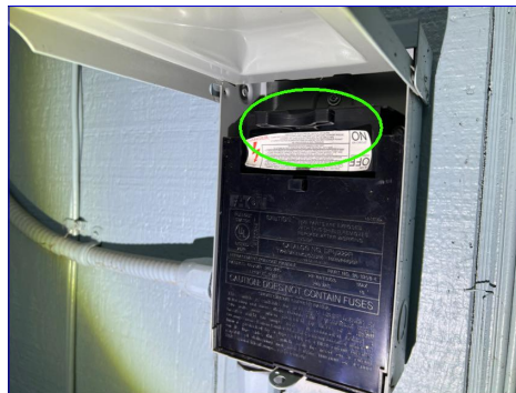
Electric service disconnect
