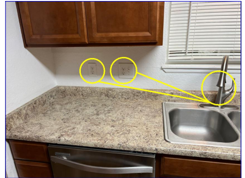
Not GFC protected (kitchen)
