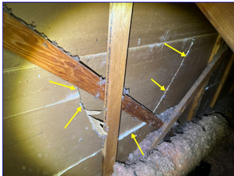
Fire separation between units is compromised
