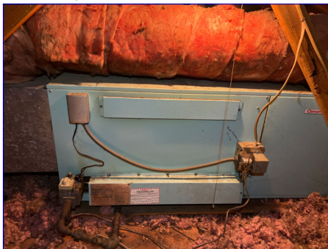
System is shut down
