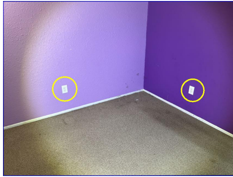
Loose receptacle(s) (Bedroom 1)
