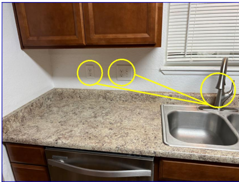
Not GFCI protected (kitchen)
