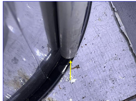
Discharge pipe not aligned with drip pan
