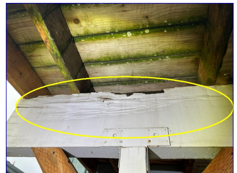
Moisture damage/wood rot
