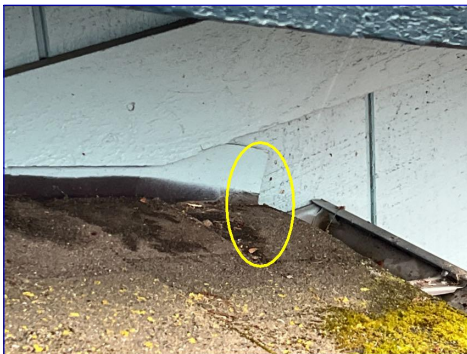
Undersized diverter flashing
