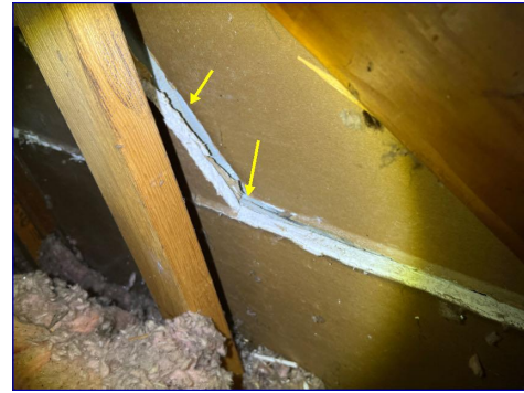
Fire separation between units is compromised
