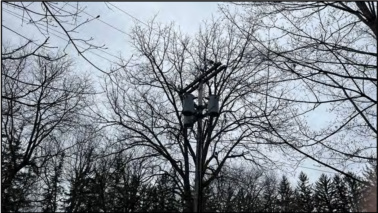
Photo 5 | View of Transformers at Southeast Corner of Addition
