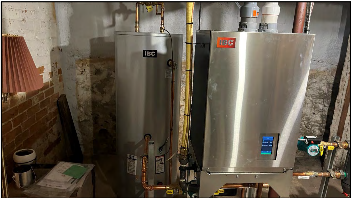
Photo 16 | View of Natural Gas Water Heater and Boiler in Original House
