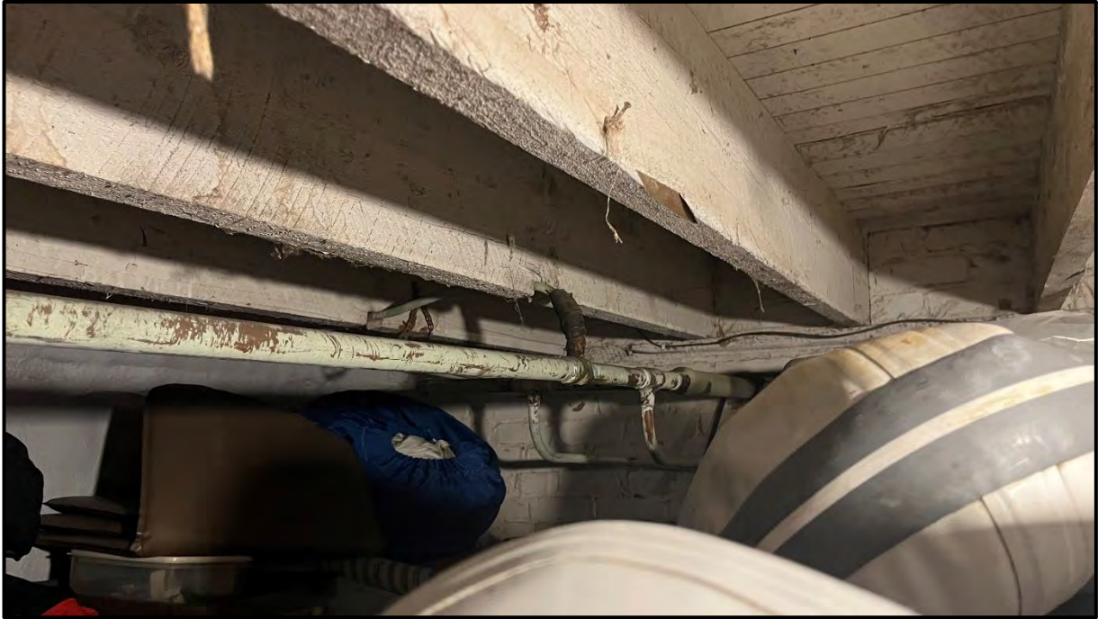
Photo 15 | View of Potential Asbestos-Containing Materials On Boiler Line In Original Basement
