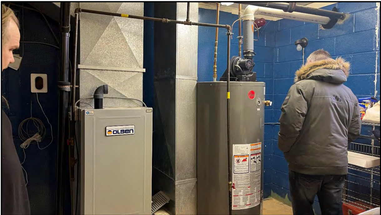
Photo 28 | View of Natural Gas Furnace and Water Heater in Basement Addition
