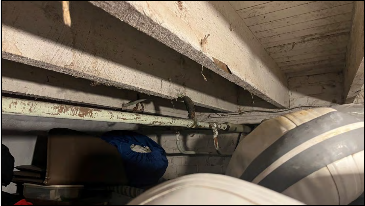
Photo 17 | View of Potentially Asbestos-Containing Materials On Boiler Line In Original Basement
