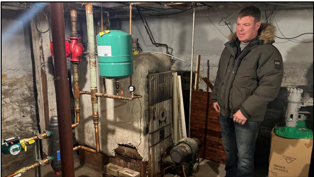
Photo 18 | View of Potentially Asbestos-Containing Materials On Historical Boiler In Original Basement
