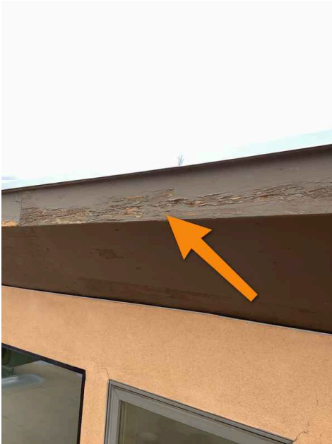
example of failing paint
