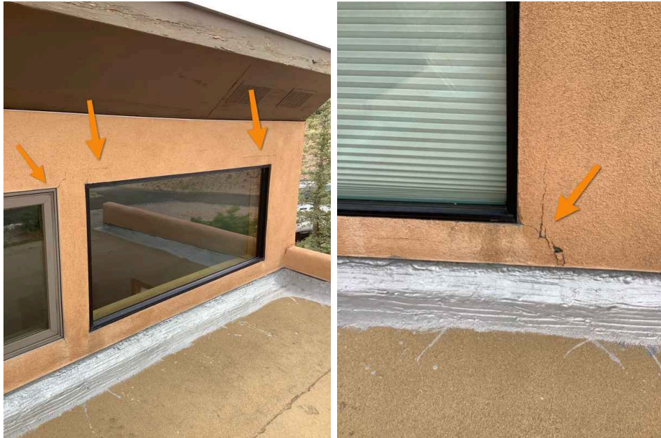
examples of stucco cracking
