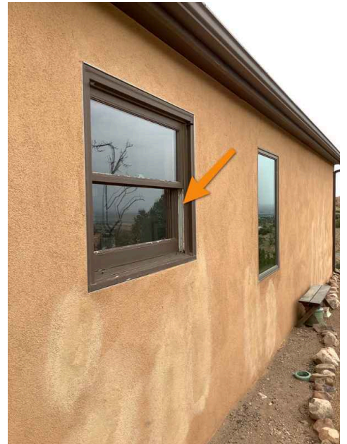
example of missing screens
