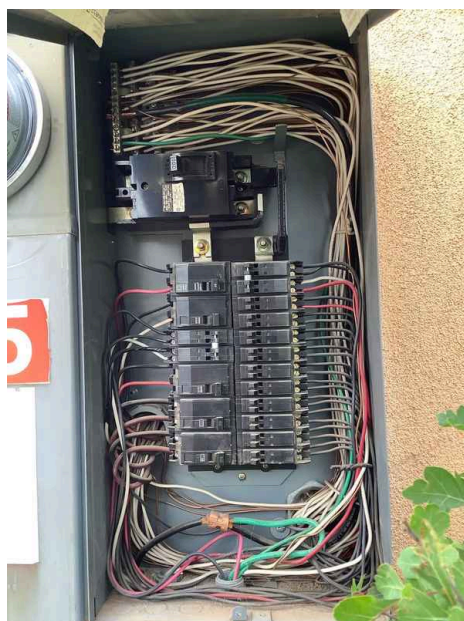
main electrical panel
