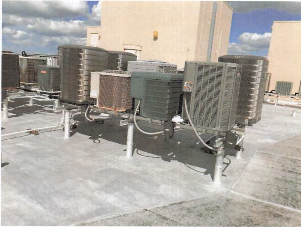
Figure 6 – A/C Condensers & Stands.
