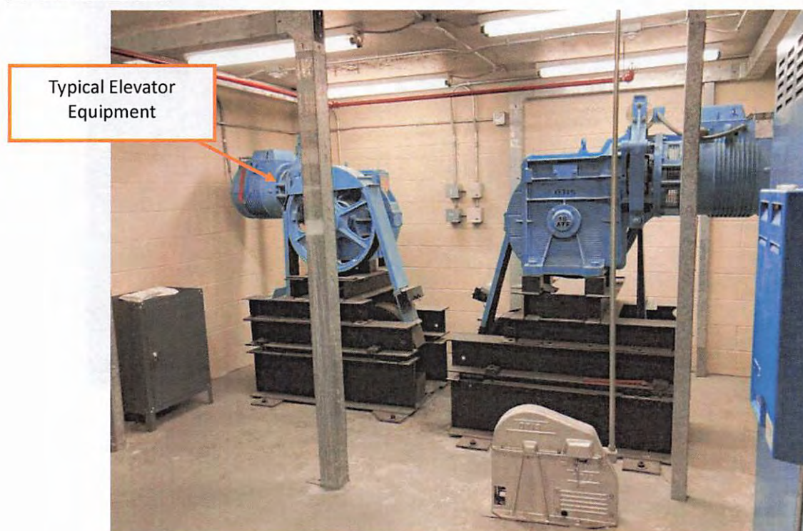
Figure 30 – Elevator Machine Room
