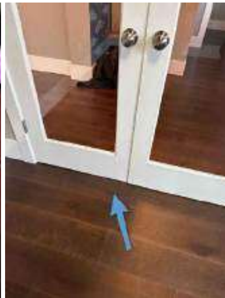
Office door rubs on the floor
