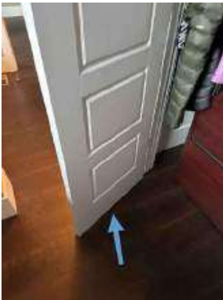
Entry closet door rubs on the floor
