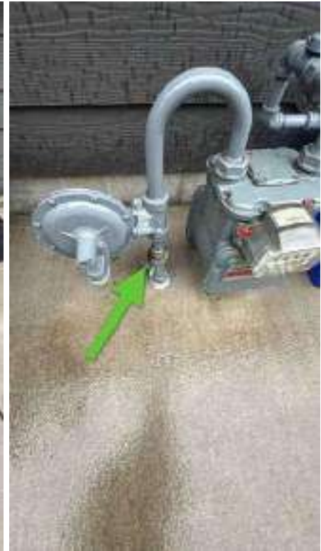
Gas Main shut off
