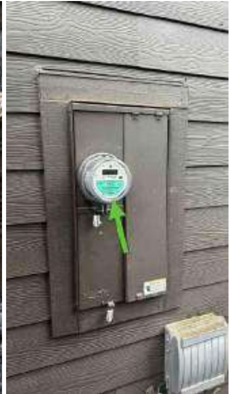
Electric Meter Right side
