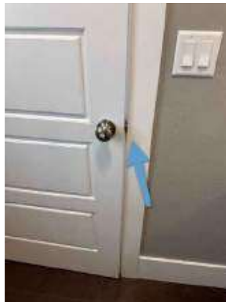
1/2 bathroom does not properly latch
