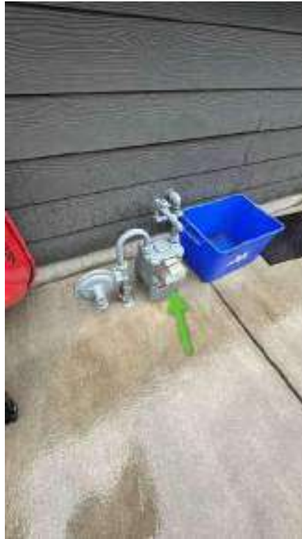
Gas Meter Left side
