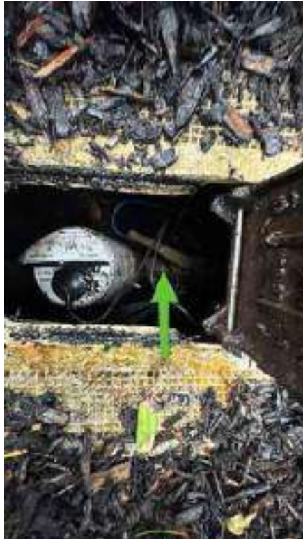
Water Main shut off
