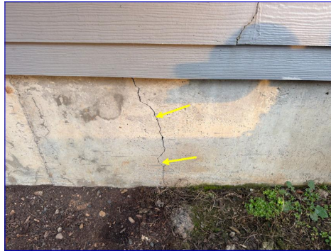
Foundation crack south
