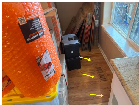
Floor is not level
