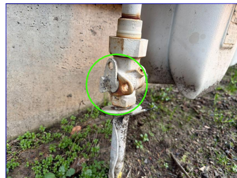
Main fuel shut off
