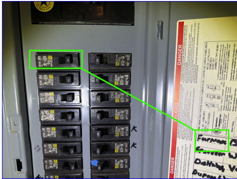
Electric service disconnect
