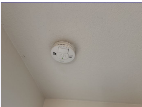
Smoke and CO alarm
