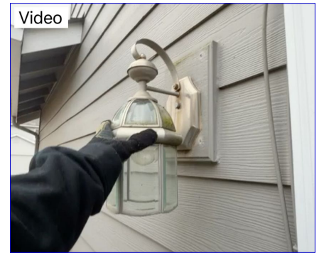
Loose exterior light fixture north
