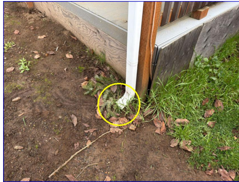
Downspout discharges at foundation
