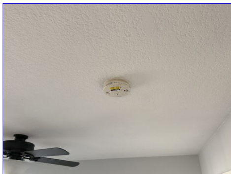
Smoke and CO alarm
