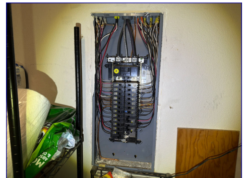
Main electric panel interior
