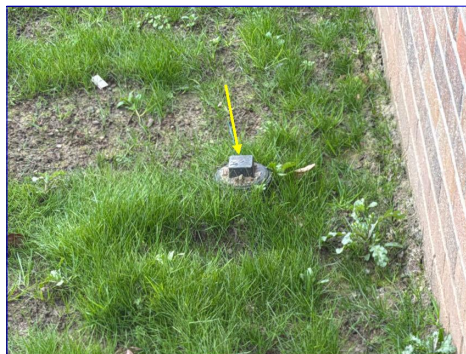
Sewer line clean out
