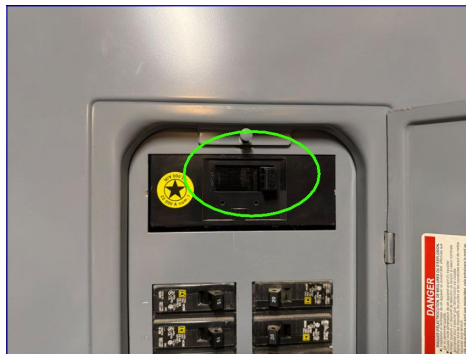
Main electric shut off
