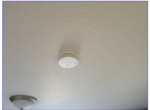
Smoke and CO alarm
