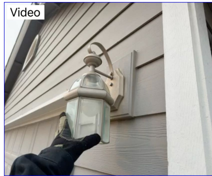
Loose exterior light fixture east
