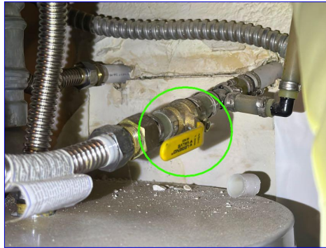
Cold water shut off
