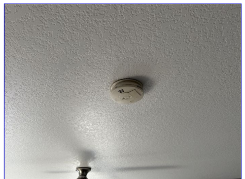
Smoke and CO alarm
