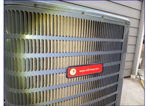
Condenser fins are dirty
