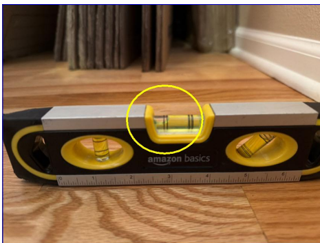
Floor is not level
