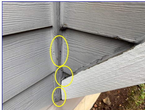
Moisture damage south
