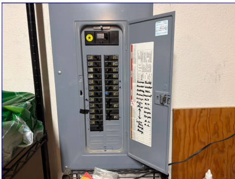
Main electric panel
