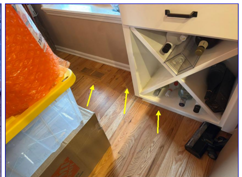
Floor is not level
