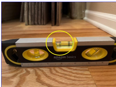
Floor is not level
