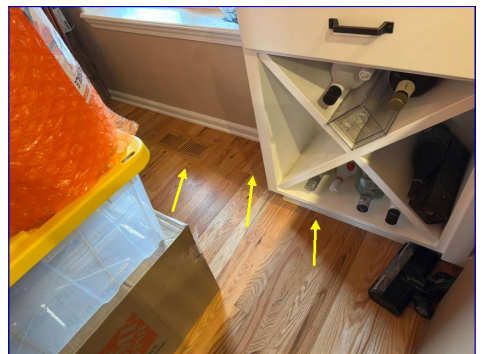
Floor is not level
