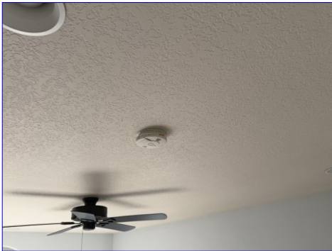
Smoke and CO alarm
