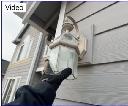
Loose exterior light fixture east
