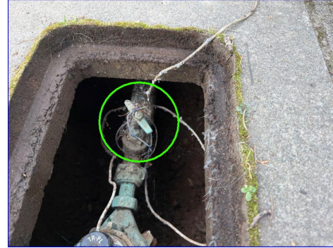
Main water shut off
