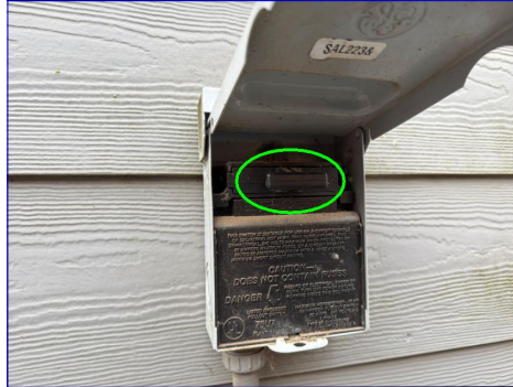
Electric service disconnect
