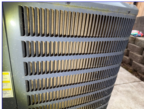
Condenser fins are dirty
