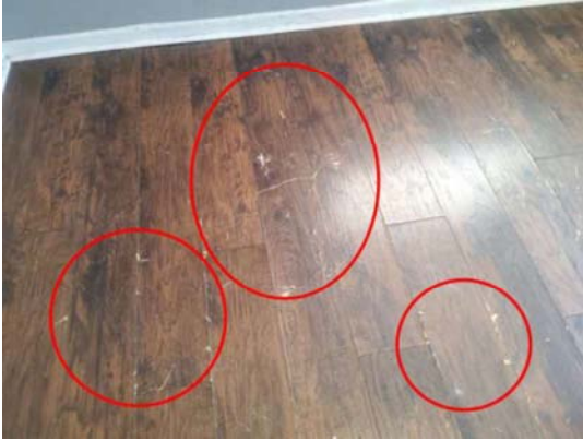
Photo 16: Laminate Floor Damage .
