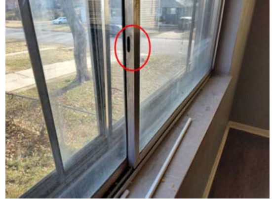
Photo 11: Windows Will Not Lock.
