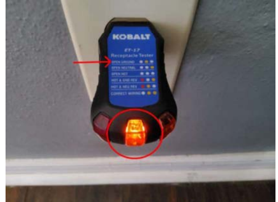
Photo 4: Ungrounded 3-prong Outlet.
