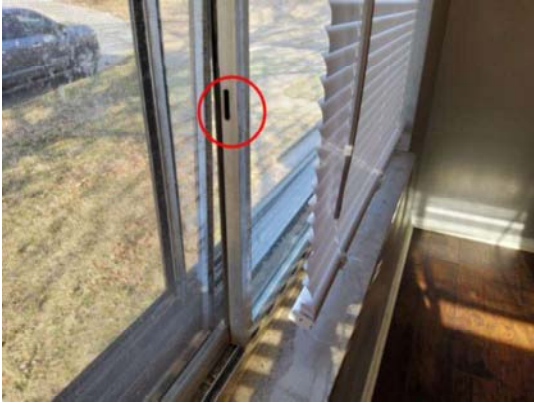
Photo 10: Windows Will Not Lock.
