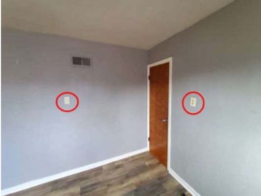
Photo 3: Ungrounded 3-prong Outlet.
