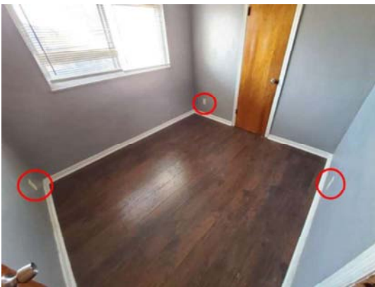
Photo 5: Ungrounded 3-prong Outlet.
