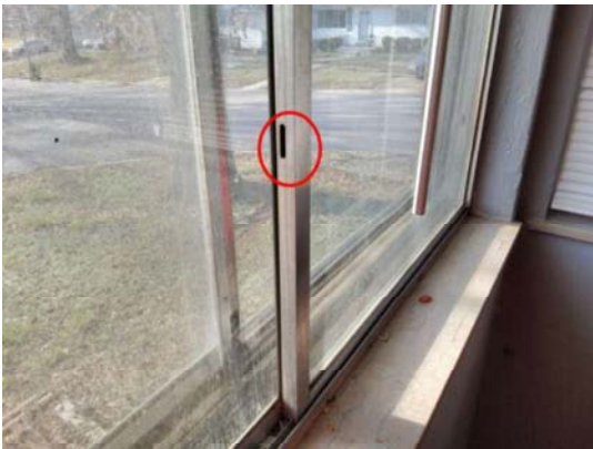
Photo 12: Windows Will Not Lock.
