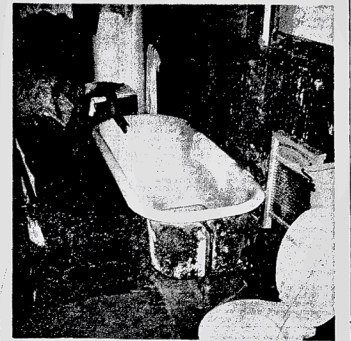
Second floor bathroom needs painting and floor repairs.
