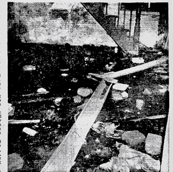
Basement room is still filthy and littered with bricks.
