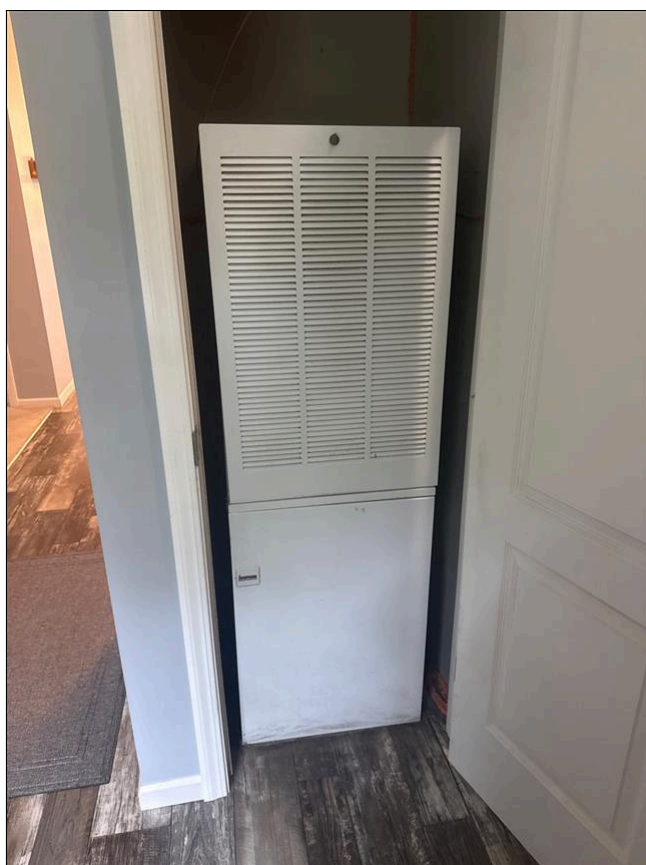
Air handler, filter located on top of unit
