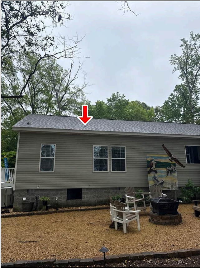
3.0 Item 1(Picture) Small nail pop on back side of roof should be monitored for future repair
