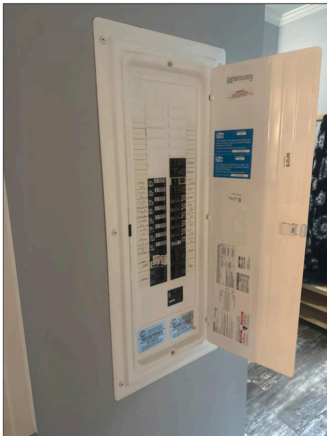
Service panel and main disconnect
