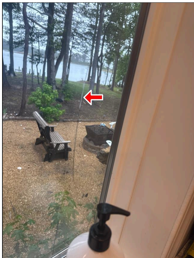
7.3 Item 1(Picture) Cracked pane
