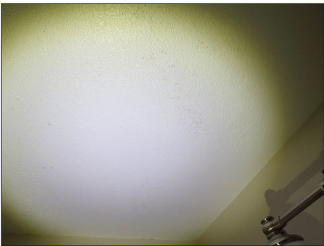
Possible microbial growth (hall bathroom)
