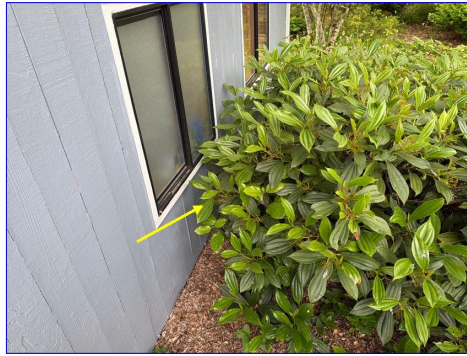
Vegetation is in contact with wall cladding
