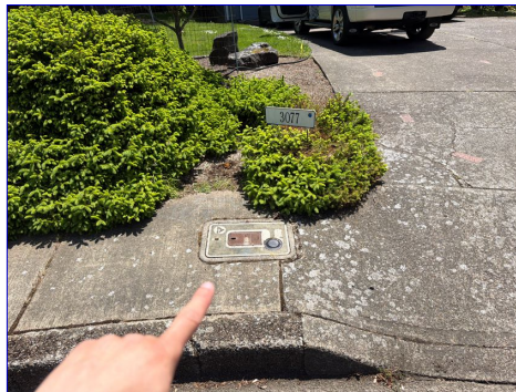
Main water shut off (water meter)
