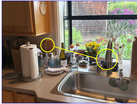
Receptacle within 6' of water source is not GFCI protected
