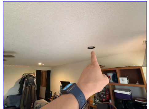
Inoperable light (Basement)
