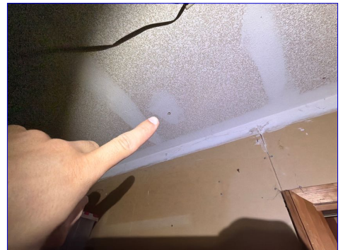
Hole in fire separation wall
