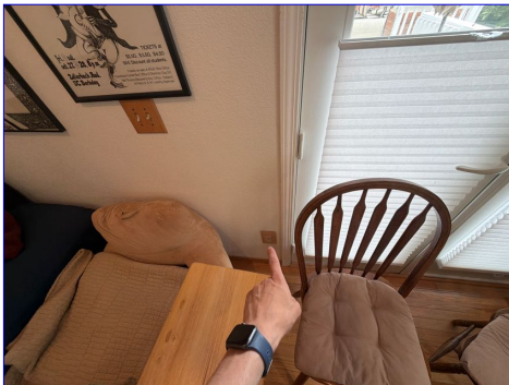
Loose receptacle in Bedroom 3
