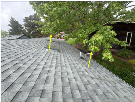
Tree limbs are too close to roof
