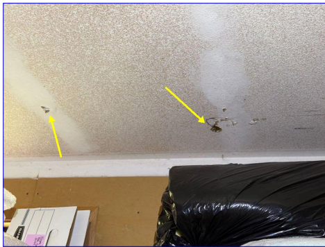
Hole in fire separation wall
