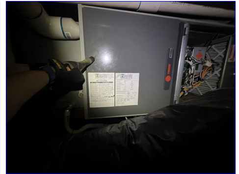
Panel is difficult to remove
