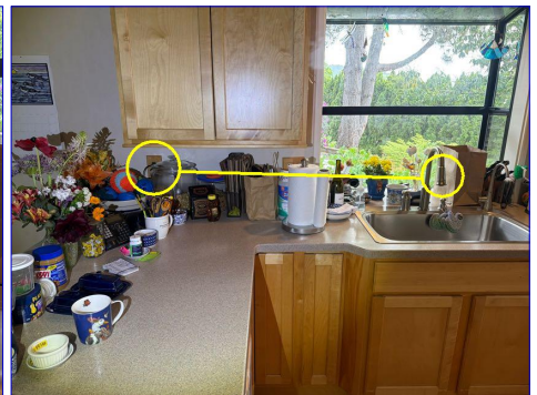
Receptacle within 6' of water source is not GFC protected
