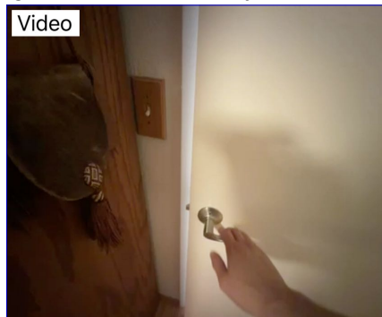
Door does not close properly
