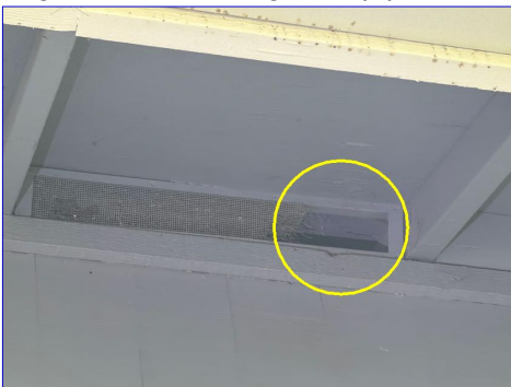
Damaged soffit vent screen (south)
