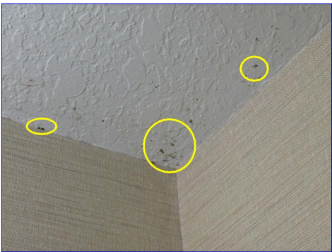
Possible microbial growth (hall bathroom)
