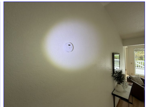
Smoke and CO alarm
