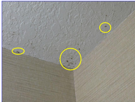
Possible microbial growth (hall bathroom)
