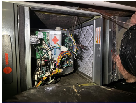
HVAC unit interior
