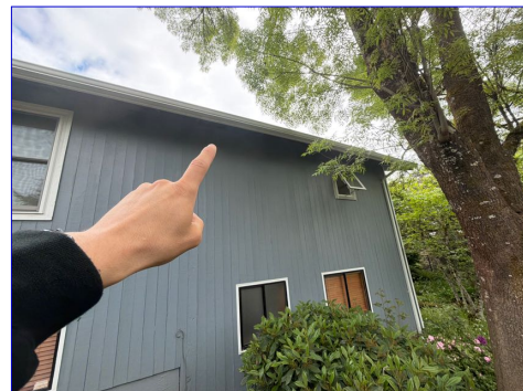
Damaged soffit vent screen (south)
