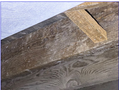
Possible microbial growth (basement closet)
