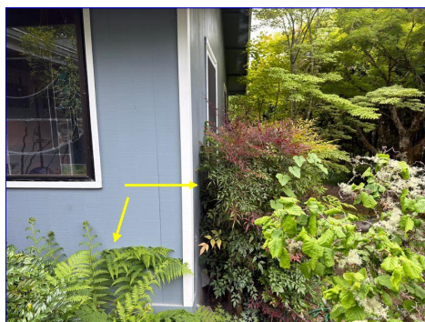
Vegetation is in contact with wall cladding
