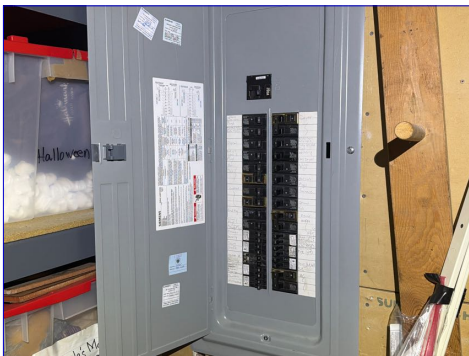
Main electric panel
