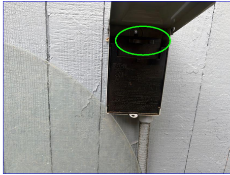
Electric service disconnect
