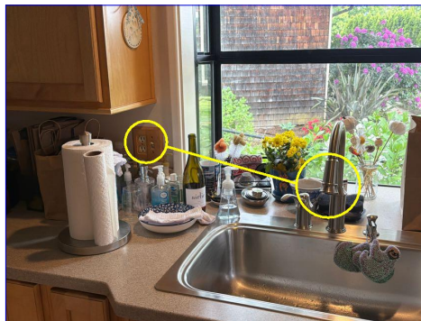
Receptacle within 6' of water source is not GFC protected
