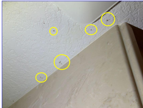
Possible microbial growth (hall bathroom)
