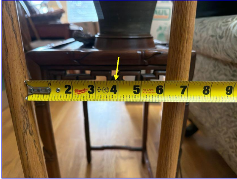
Balusters spacing exceeds 4"
