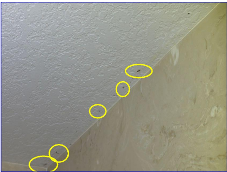
Possible microbial growth (hall bathroom)
