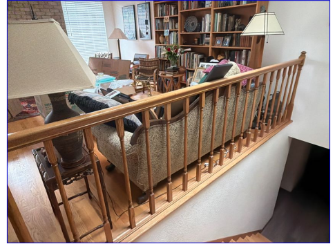
Balusters spacing exceeds 4"
