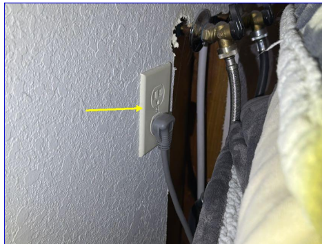
Washing machine receptacle is not GFCI protected
