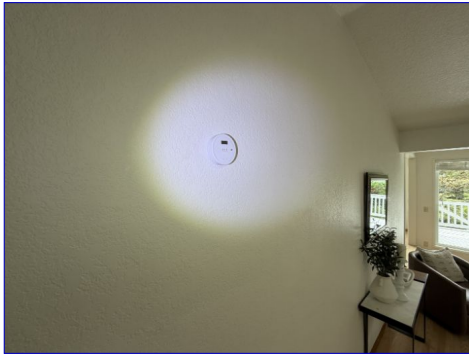
Smoke and CO alarm
