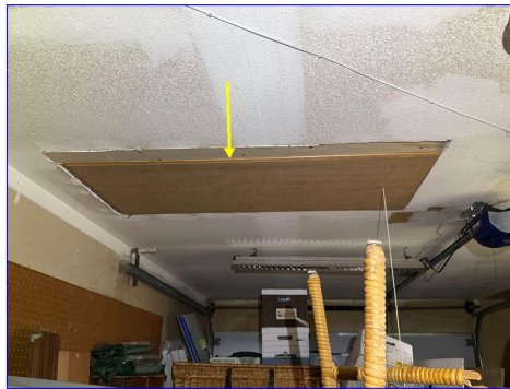
Attic access is flammable
