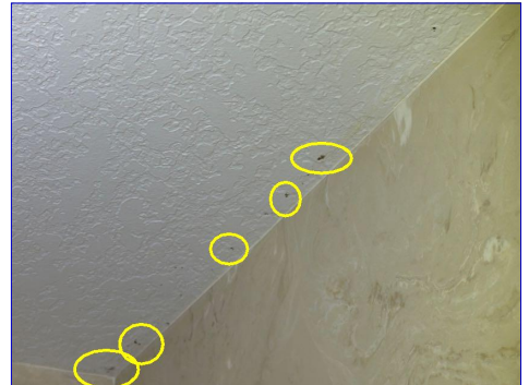
Possible microbial growth (hall bathroom)
