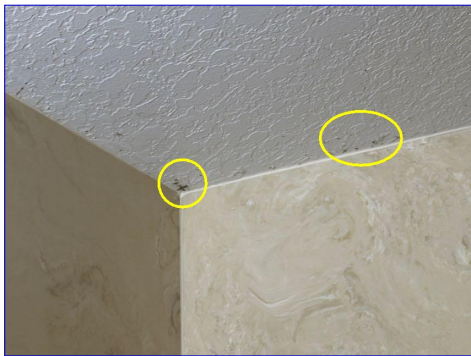
Possible microbial growth (hall bathroom)
