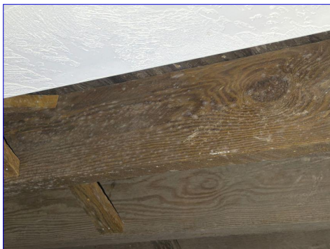
Possible microbial growth (basement closet)
