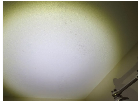
Possible microbial growth (hall bathroom)
