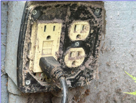
Lint covering exterior receptacle (front)
