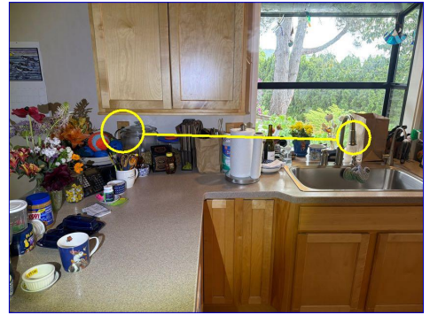
Receptacle within 6' of water source is not GFCI protected
