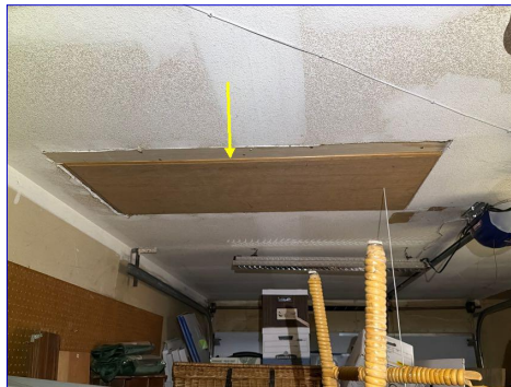
Attic acces is flammable
