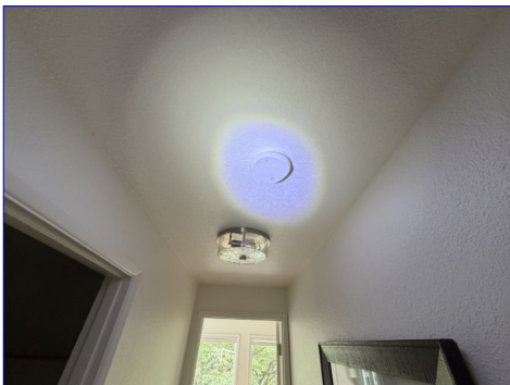
Smoke and CO alarm
