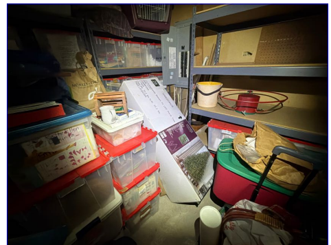
Pathway blocked to panel
