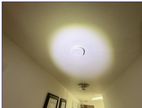
Smoke and CO alarm
