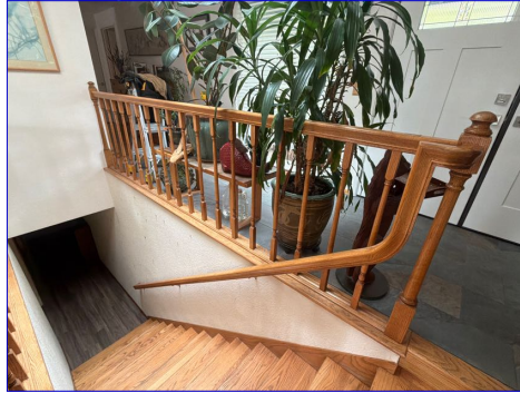
Balusters spacing exceeds 4"
