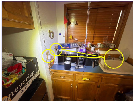
Basement receptacles within 6' of water source are not GFCI protected
