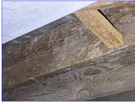
Possible microbial growth (basement closet)
