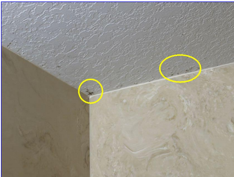
Possible microbial growth (hall bathroom)
