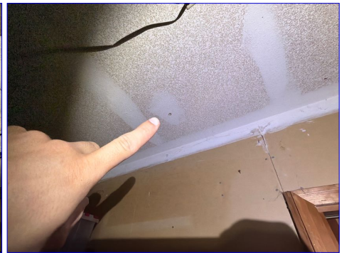
Hole in fire separation wall
