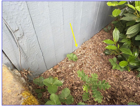
Soil is in contact with wall cladding (south)
