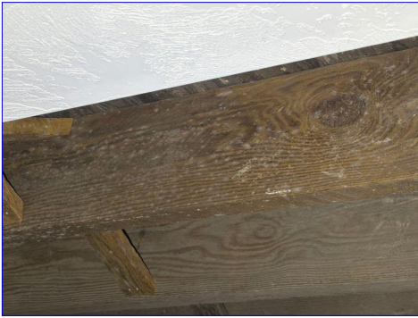
Possible microbial growth (basement closet)
