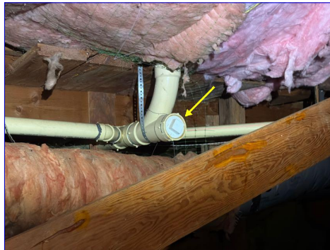
Sewer line clean out
