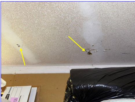
Hole in fire separation wall
