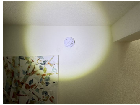
Smoke and CO alarm
