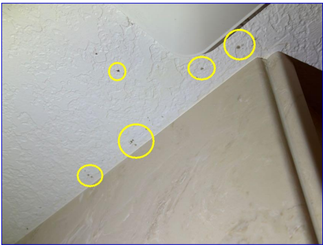
Possible microbial growth (hall bathroom)
