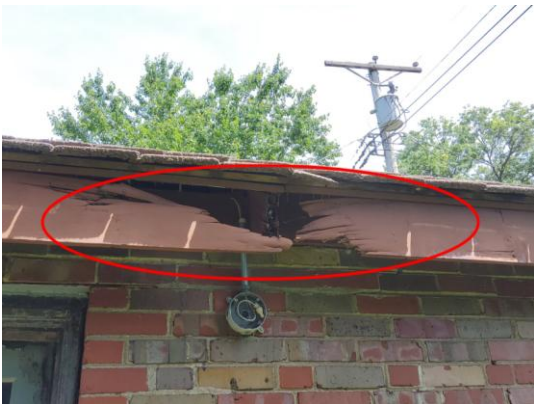
Photo 18: Fascia Substantial Rot.
