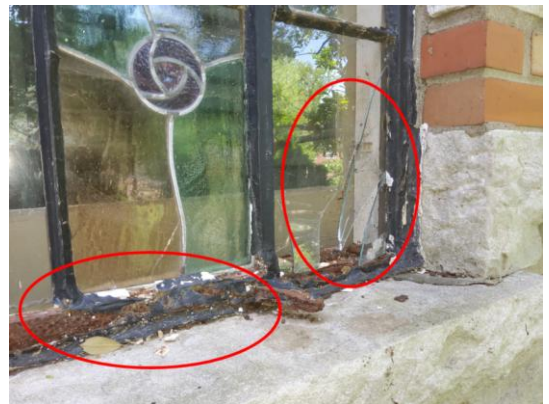
Photo 19: Dilapidated Windows, Replace.
