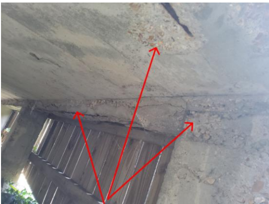
Photo 12: Porch Masonry Spalling.
