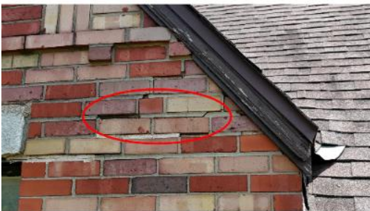
Photo 14: Brick Localized Pointing.
