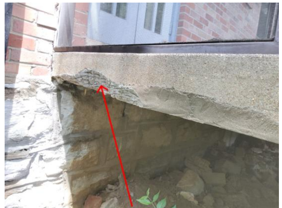
Photo 13: Porch Masonry Spalling.
