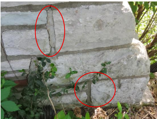
Photo 3: Cracks Moderate - Settling.
