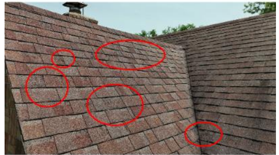
Photo 8: Roofing Nearing End of Life Cycle.
