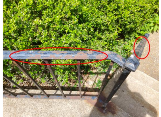
Photo 11: Steel Railing Paint.
