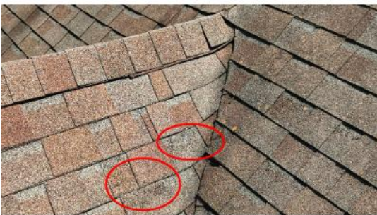
Photo 9: Roofing Nearing End of Life Cycle.
