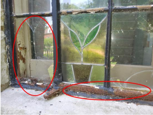
Photo 22: Dilapidated Windows, Replace.
