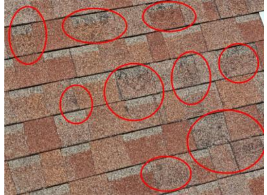
Photo 6: Roofing Nearing End of Life Cycle.
