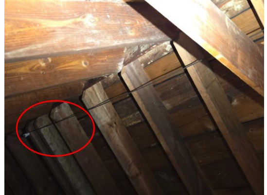
Photo 24: Knob & Tube Wiring.
