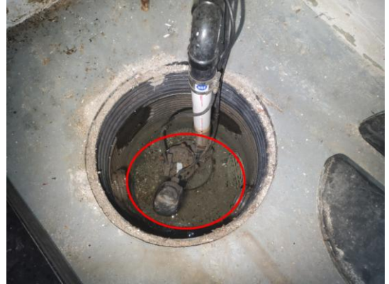
Photo 29: Sump Pump Inoperative.
