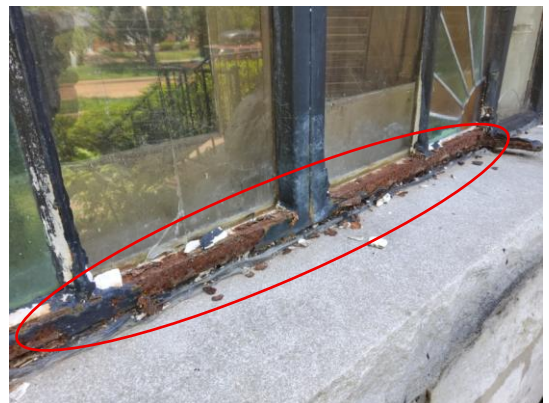
Photo 21: Dilapidated Windows, Replace.
