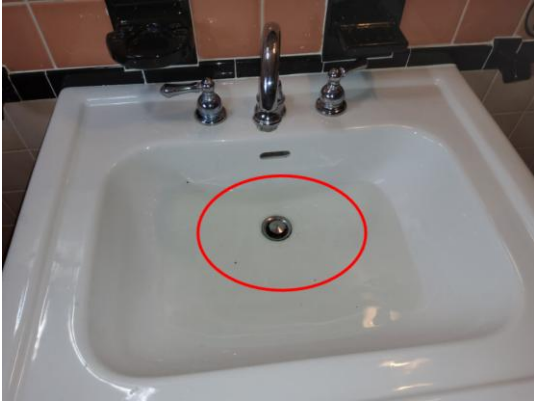
Photo 28: Sink Drains Slow.
