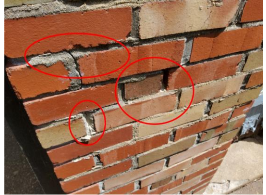
Photo 17: Brick Localized Pointing.
