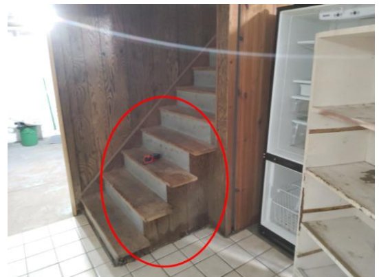
Photo 42: Stair Railing Needed.
