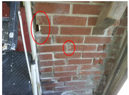
Photo 15: Brick Localized Pointing.
