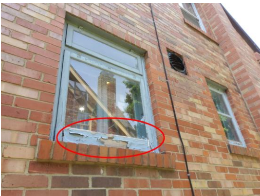
Photo 20: Dilapidated Windows, Replace.
