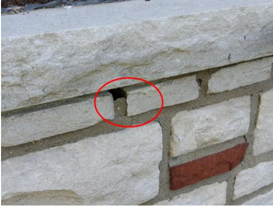
Photo 16: Brick Localized Pointing.
