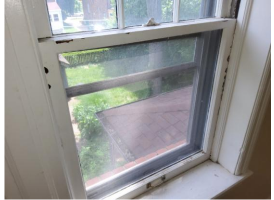
Photo 44: Old Windows - Mild Disrepair.
