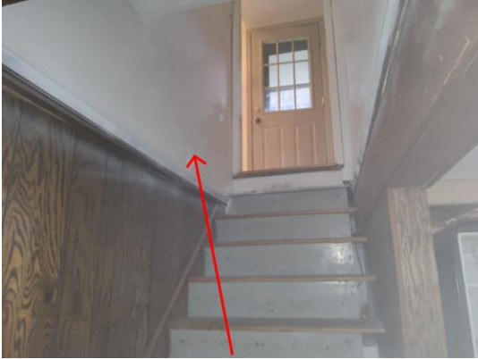
Photo 43: Stair Handrail Needed.
