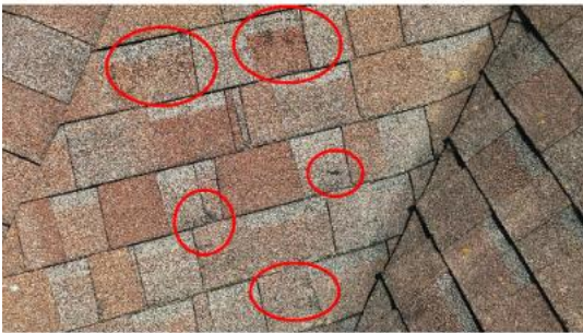
Photo 7: Roofing Nearing End of Life Cycle.
