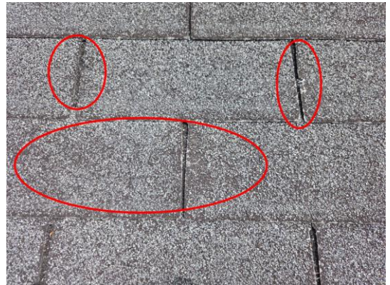
Photo 11: Roofing Nearing End of Life Cycle.
