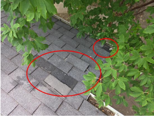
Photo 8: Roofing Nearing End of Life Cycle.
