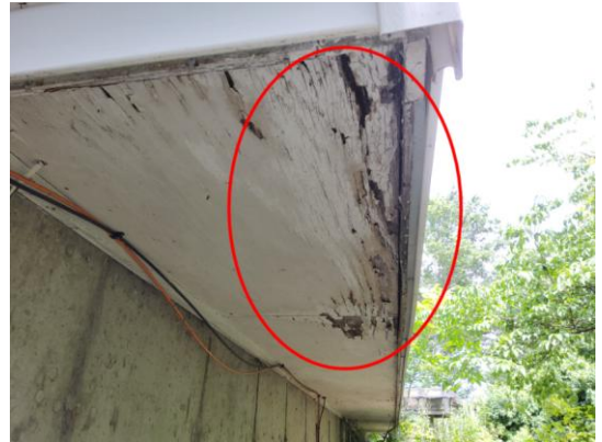
Photo 15: Bay Areas Pressboard Underneath.
