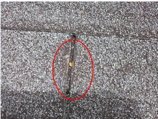
Photo 4: Roofing Nearing End of Life Cycle.
