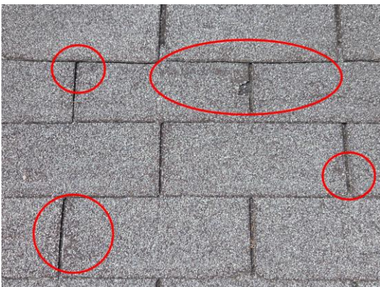
Photo 12: Roofing Nearing End of Life Cycle.
