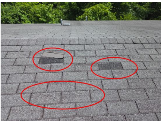
Photo 6: Roofing Nearing End of Life Cycle.
