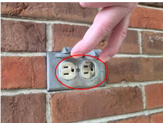
Photo 23: GFCI None Present.
