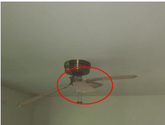
Photo 27: Ceiling Fan Inoperative.
