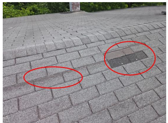
Photo 7: Roofing Nearing End of Life Cycle.
