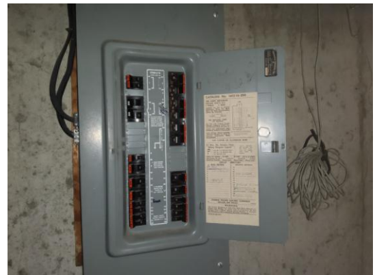
Photo 28: Federal Pacific Panel Obsolete.
