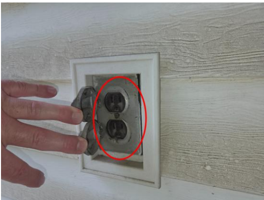
Photo 21: GFCI None Present.
