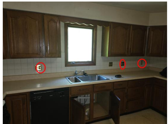
Photo 22: GFCI None Present.
