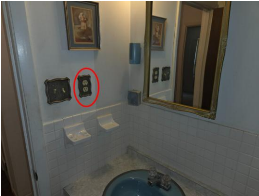
Photo 19: GFCI None Present.
