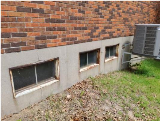
Photo 14: Basement Windows Neglected.
