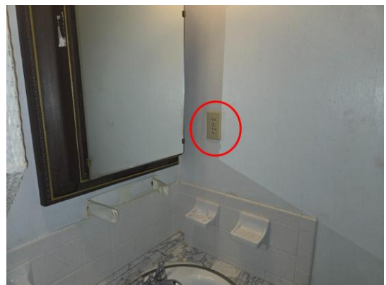
Photo 24: GFCI None Present.
