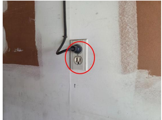
Photo 20: GFCI None Present.
