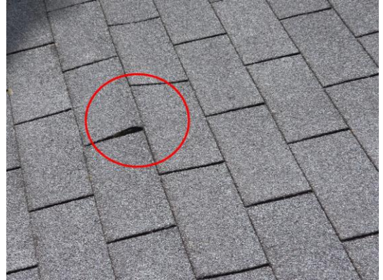
Photo 3: Roofing Nearing End of Life Cycle.
