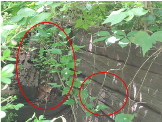
Photo 18: Significant Movement and Rot.
