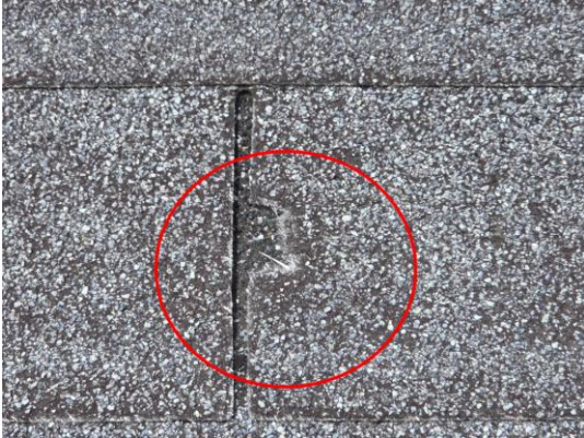
Photo 2: Roofing Nearing End of Life Cycle.
