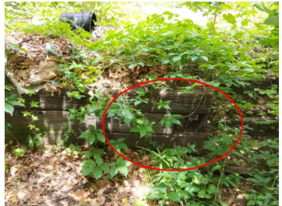
Photo 17: Significant Movement and Rot.
