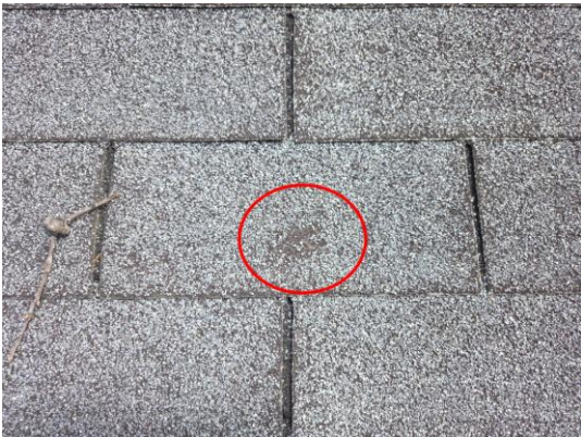
Photo 10: Roofing Nearing End of Life Cycle.
