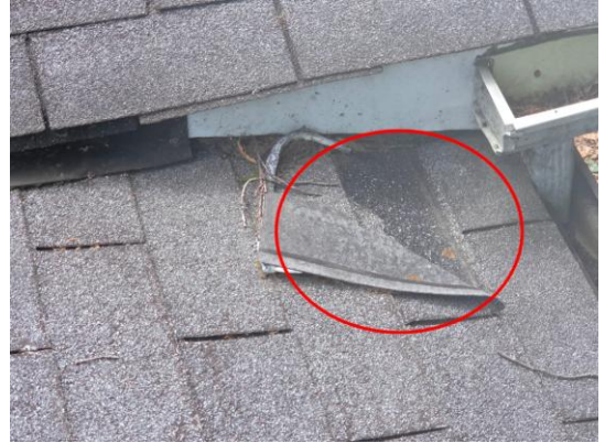
Photo 9: Roofing Nearing End of Life Cycle.
