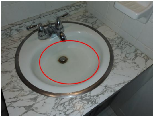
Photo 31: Sink Drains Slow.
