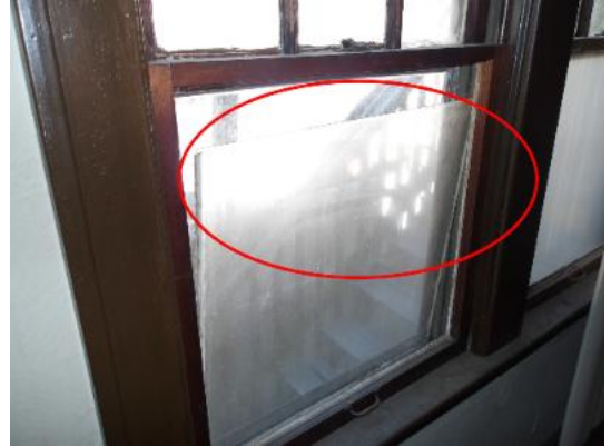
Photo 37: Old Windows - Mild Disrepair.
