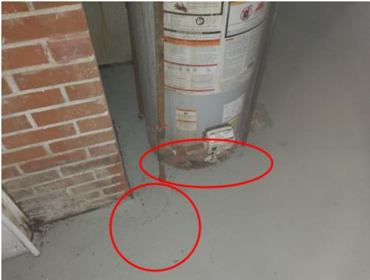
Photo 17: Active Tank Leak.
