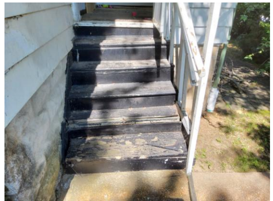
Photo 7: Wood Stairs Dilapidated .
