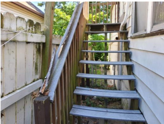
Photo 8: Wood Stairs Dilapidated .
