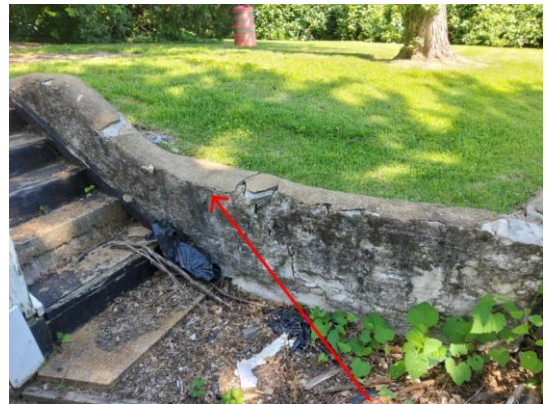
Photo 13: Retaining Wall Slight Movement.
