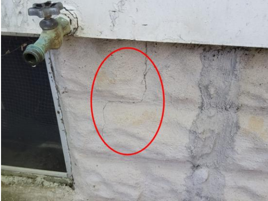
Photo 1: Cracks Minor - Settling.
