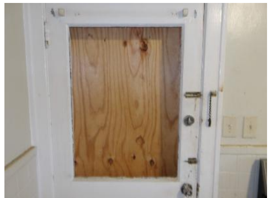
Photo 35: Old Windows - Mild Disrepair.
