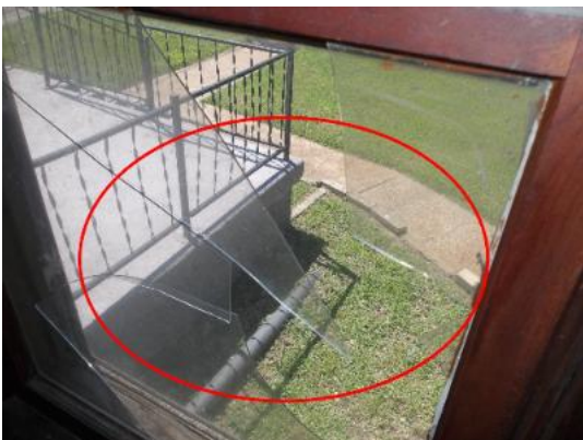
Photo 34: Old Windows - Mild Disrepair.
