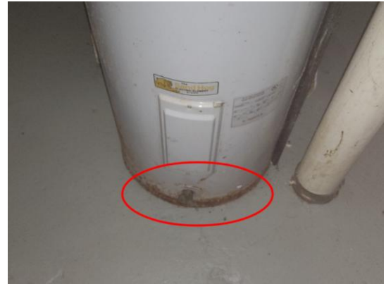
Photo 18: Prior Leak Evidence - Base Corrosion.
