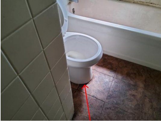
Photo 23: Toilet Loose on Base.
