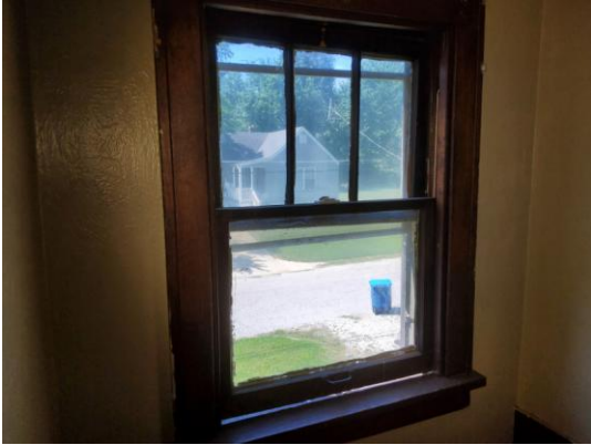
Photo 36: Old Windows - Mild Disrepair.
