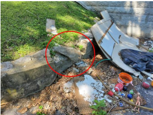
Photo 12: Retaining Wall Slight Movement.
