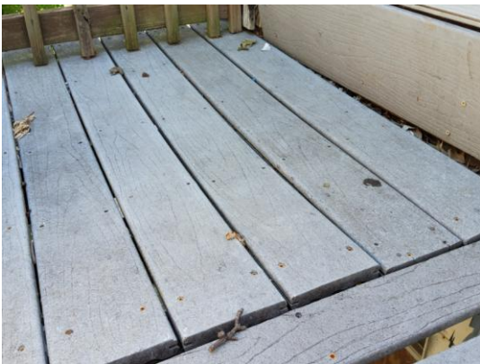
Photo 6: Wood Stairs Dilapidated .
