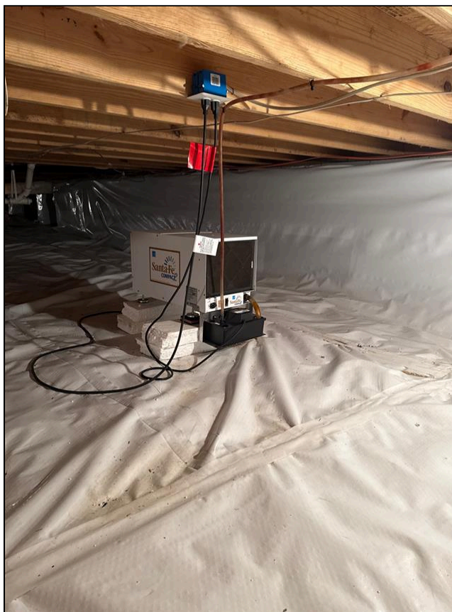
Dehumidifier in crawlspace, functional
