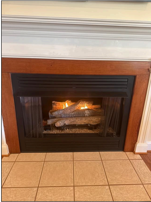
Gas logs, in operation
