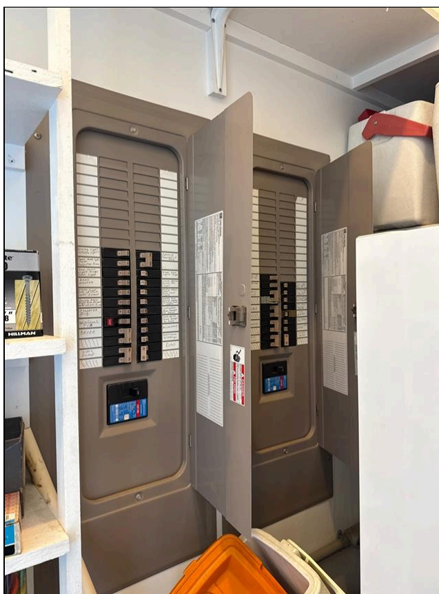
Service panels and main disconnects
