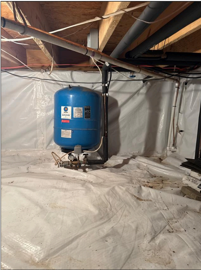
Well system equipment in crawlspace
