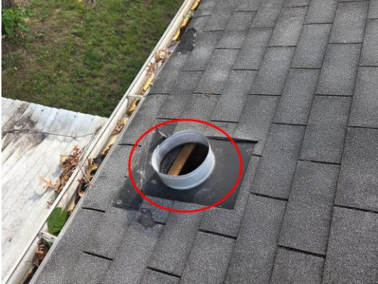
Photo 4: Roof Vent Cap Missing.
