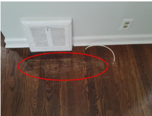
Photo 32: Wood Floor Damage.
