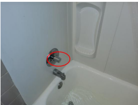
Photo 26: Shower Valve Stops Missing.
