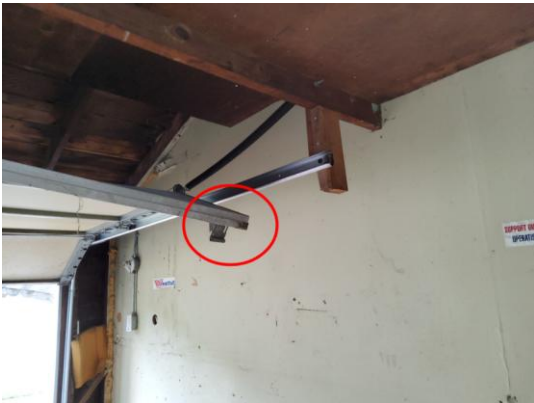
Photo 11: Overhead Door Minor Damage.
