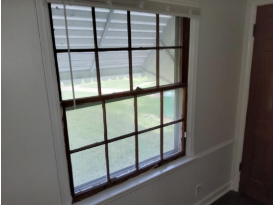
Photo 28: Old Windows - Mild Disrepair.
