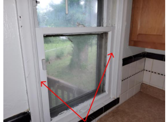
Photo 29: Window Painted Shut.
