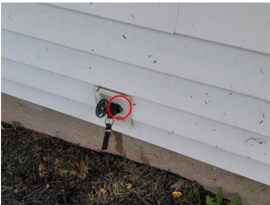
Photo 24: Hose Bib Loose .
