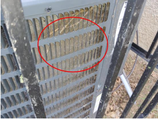
Photo 20: Outdoor Unit Dirty.
