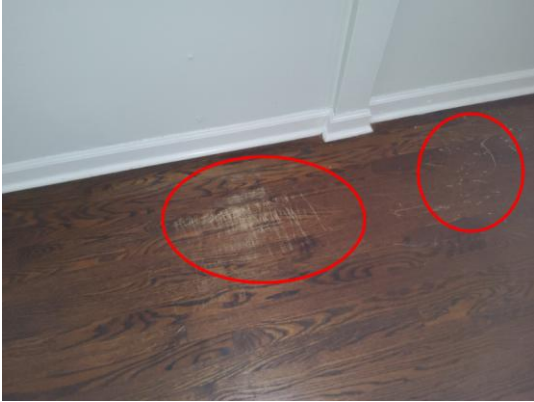
Photo 34: Wood Floor Damage.
