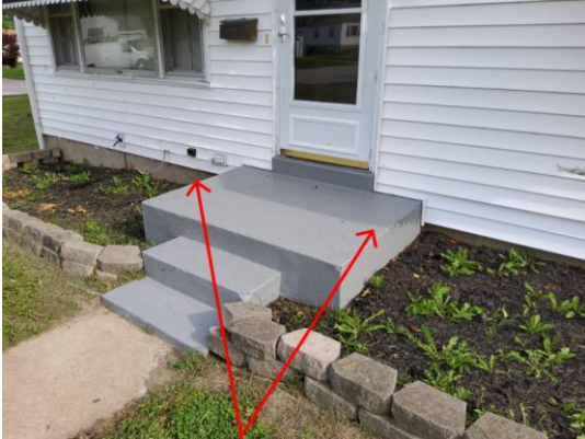
Photo 9: Porch Railing Needed.
