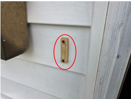
Photo 37: Door Bell Inoperative.
