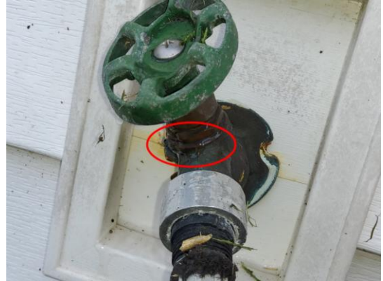
Photo 23: Hose Bibb Leaky.
