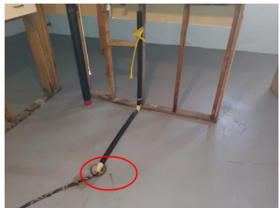
Photo 27: Waste Standpipe Routed to Floor Drain.
