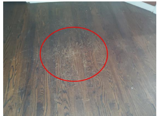
Photo 31: Wood Floor Damage.
