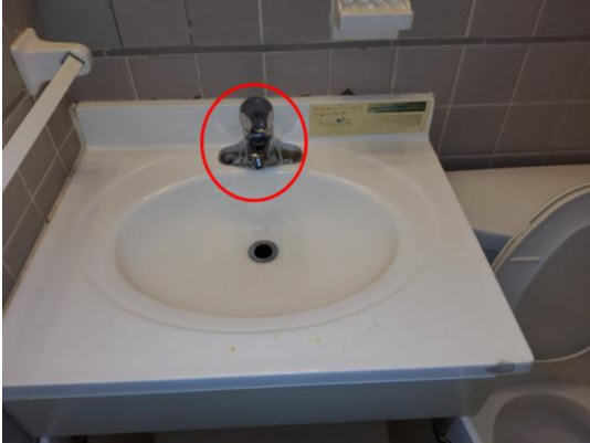
Photo 22: Hot/Cold Supply Reversed.
