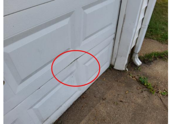
Photo 10: Overhead Door Minor Damage.
