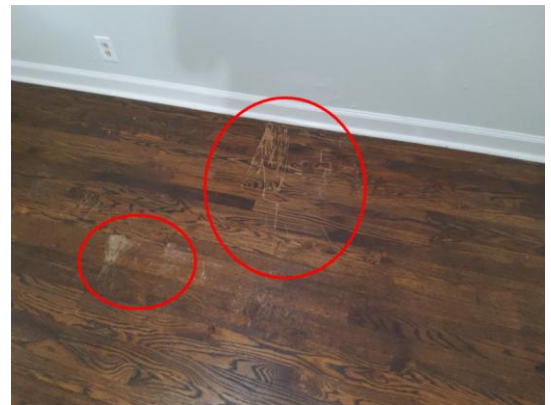
Photo 33: Wood Floor Damage.
