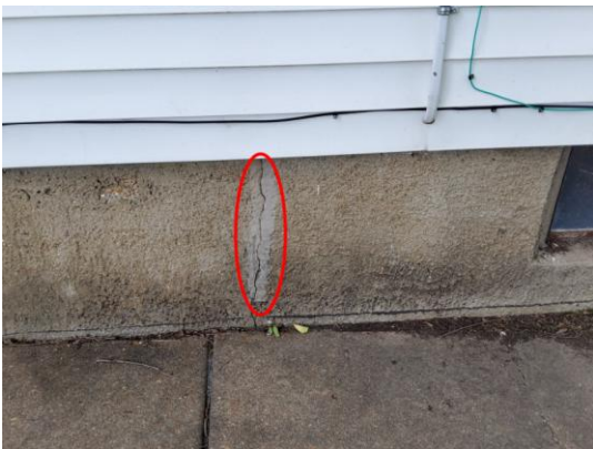
Photo 3: Cracks Minor - Shrinkage.
