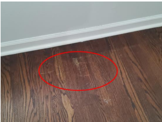
Photo 30: Wood Floor Damage.
