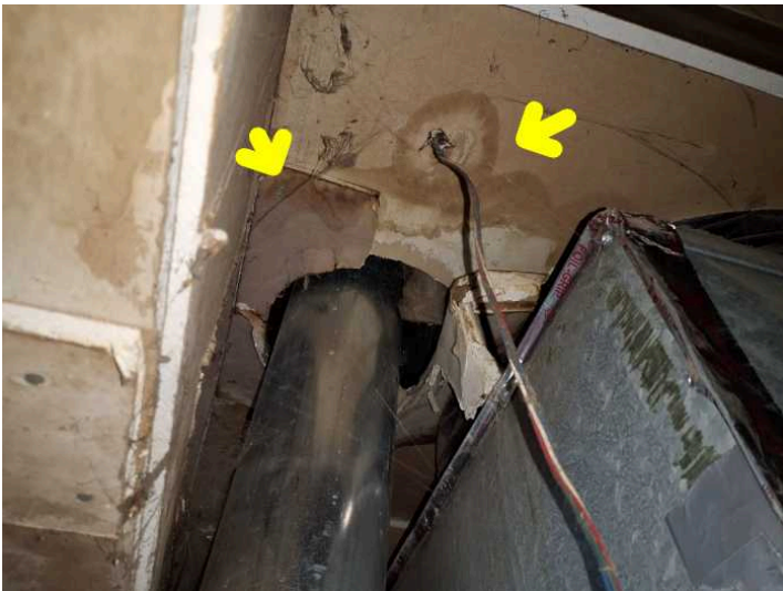
There are moisture stains on the ceiling at the vent pipe which should be explained or further explored. It could indicate the roof vent flashing is not properly sealed.
