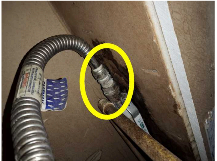
There is a leak at the water connector on the inlet side of the gas water heater, which should be repaired by a qualified tradesperson.
