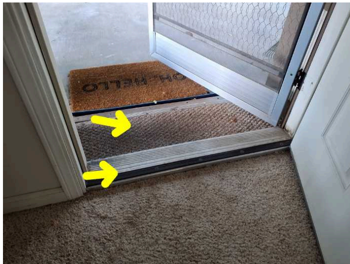
There is damage to the threshold that should be evaluated by a qualified specialist and serviced as necessary.
