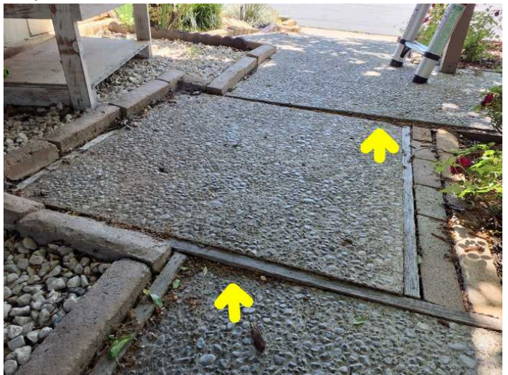
There are one or more offsets in the walkways or patio that could prove to be trip-hazards.
