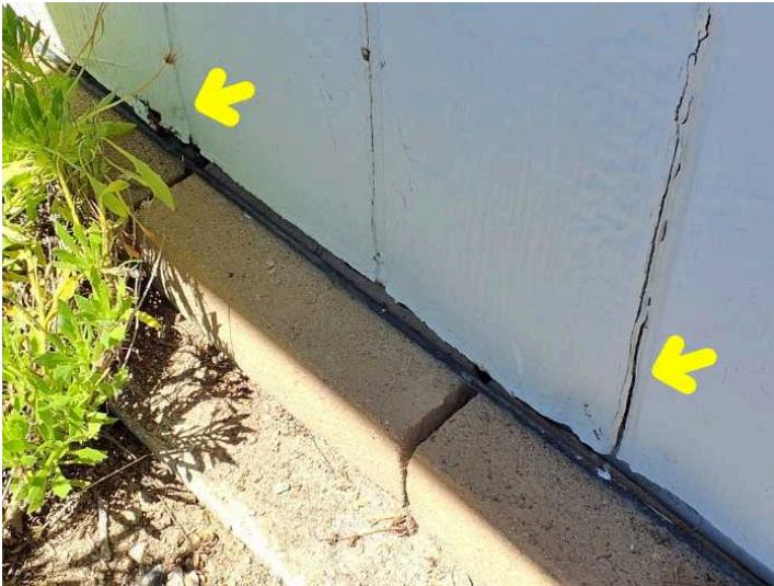
Portions of the siding have dry rot or are moisture damaged, and should be evaluated by a pest inspector.
