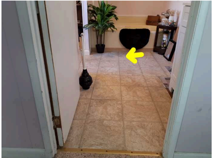
The floor is out of level. We can elaborate, but this condition should be evaluated by a qualified tradesperson.
