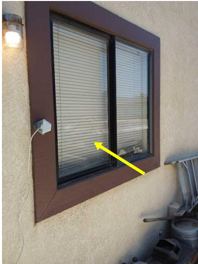
A window screen is missing, which you may wish to have replaced.
