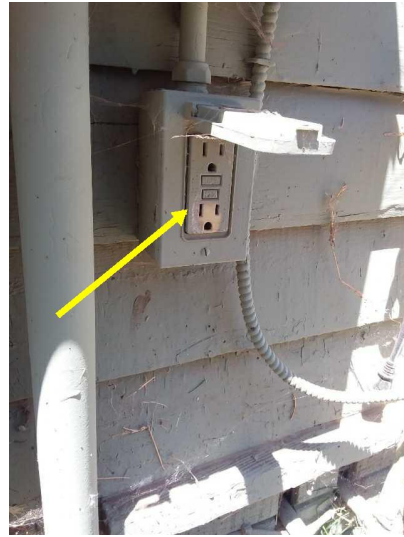
A ground-fault protected outlet in the rear of the house does not trip on test, and should be serviced.
