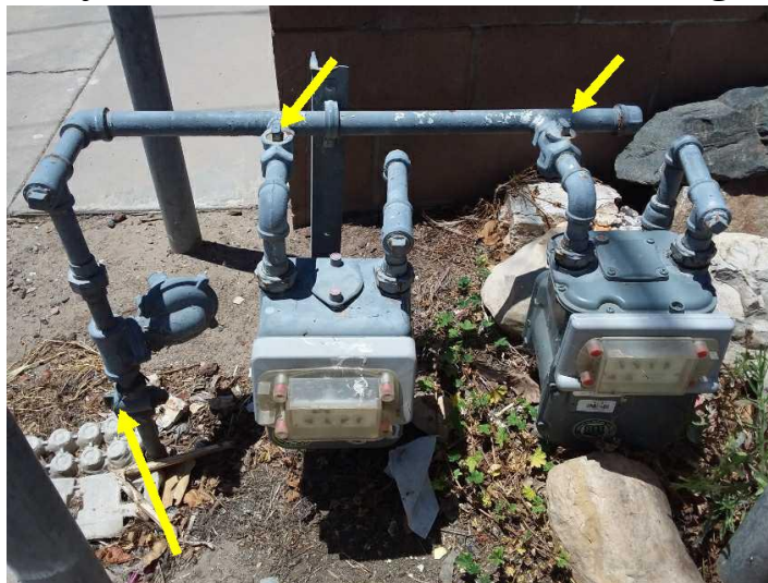
The gas main shut-off is located on left side of the home at 630 unit B.
