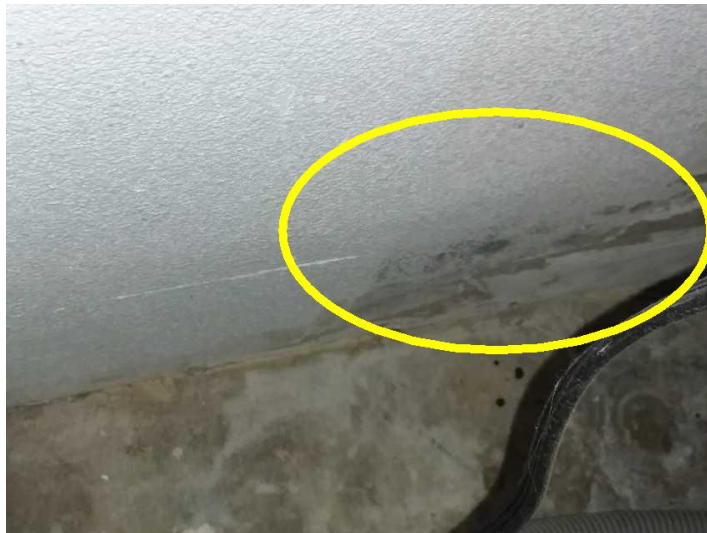
There is a mold-like substance that we will point out, which should be evaluated by a specialist. All molds flourish in a damp environment and many are commonplace, but some are toxic and represent a health threat.
