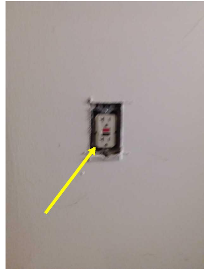
One or more outlet covers is missing and should be installed.
