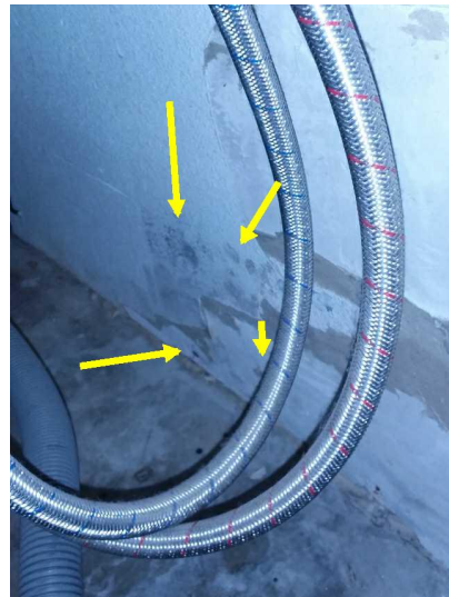
There is a mold-like substance that we will point out, which should be evaluated by a specialist. All molds flourish in a damp environment and many are commonplace, but some are toxic and represent a health threat.
