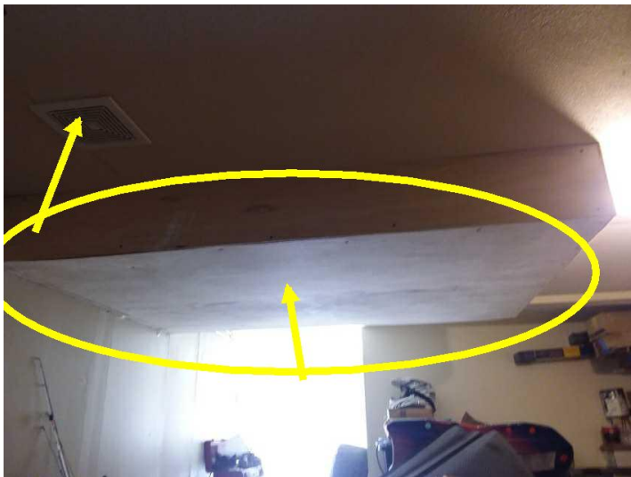
The voids in the ceiling firewall must be repaired, in order to maintain the necessary firewall separation between the garage and the residence.
