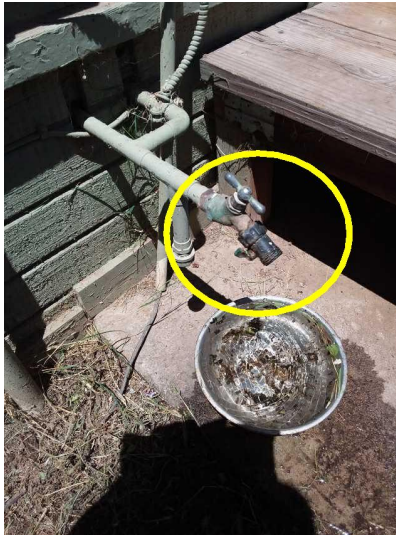
A hose bib at the rear leaks and should be serviced.
