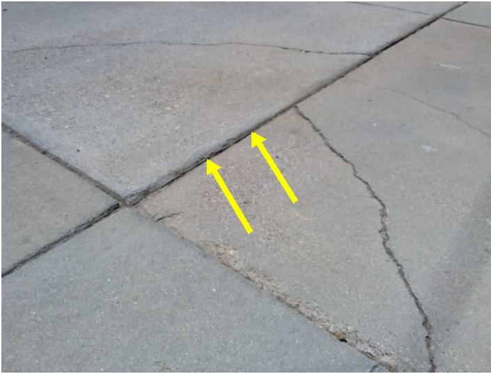
There is one or more offsets in the driveway that could prove to be trip-hazards.
