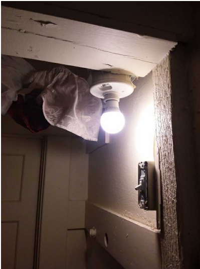
The closet employs a light bulb that should have a cover.
