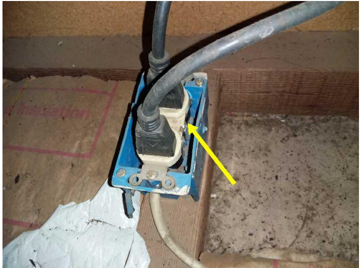
One or more outlets is missing a cover which should be installed.
