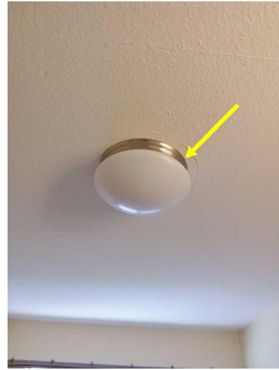
A ceiling light does not respond and should be serviced.
