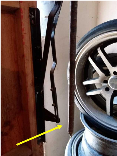
A door spring is missing or broken, and should be replaced.
