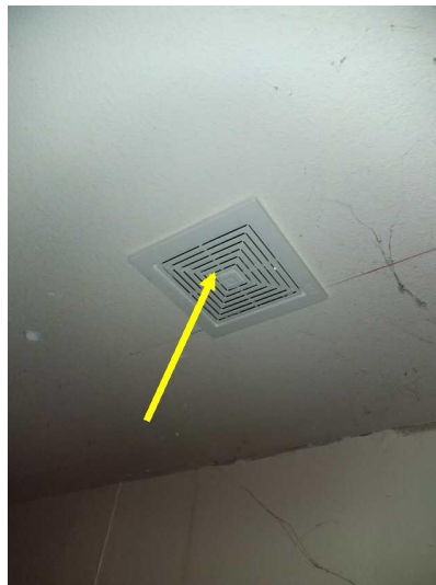
The voids in the ceiling firewall must be repaired, in order to maintain the necessary firewall separation between the garage and the residence.
