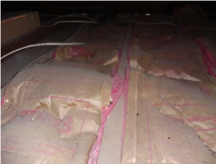
Some paper-faced, batt, insulation in the attic has been installed upside down. This is of no serious consequence, but the paper-face is intended to be installed toward the heated area or inside of the residence.
