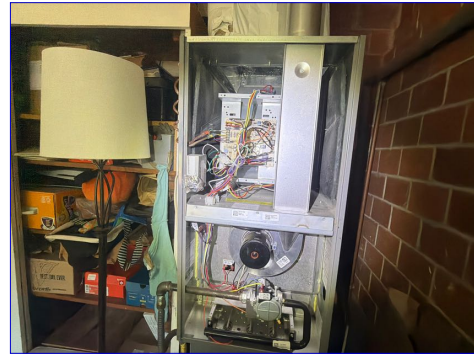
HVAC unit interior
