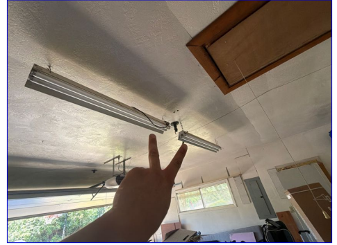
Inoperable/not plugged in light fixtures (garage)
