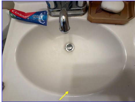
Missing overflow drain
