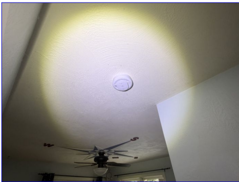
Smoke and CO alarm
