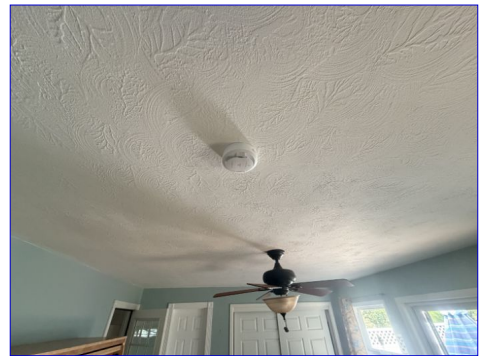
Smoke and CO alarm
