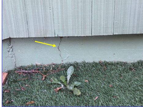
Foundation crack (north)
