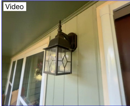
Loose exterior light fixture (front)
