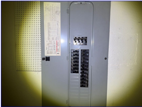
Main electric panel
