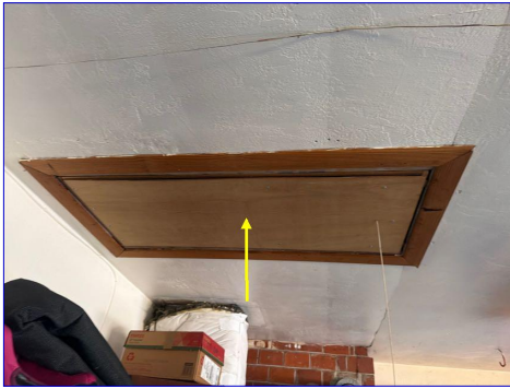
Attic access is flammable
