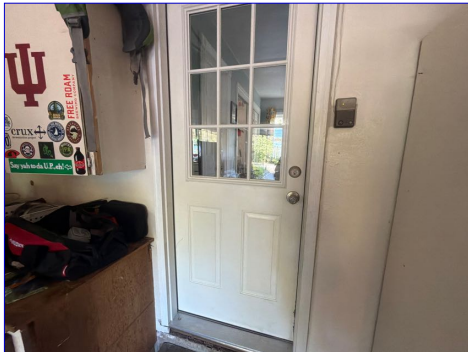
Door does not automatically close
