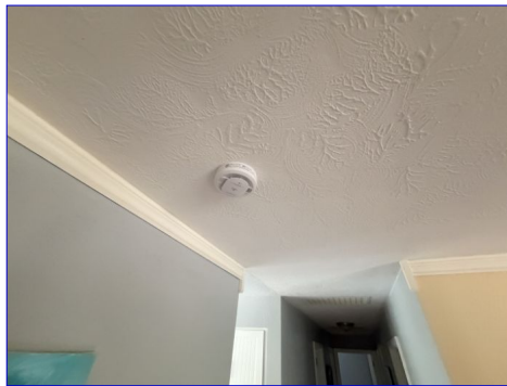
Smoke and CO alarm
