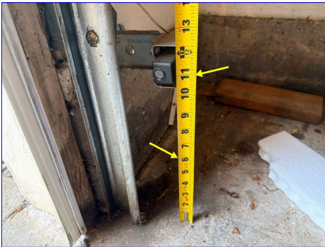
Photo eye sensor is too high
