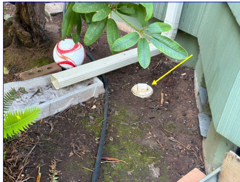
Sewer line clean out
