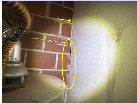
Hole in fire separation wall
