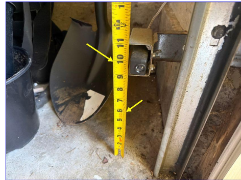
Photo eye sensor is too high
