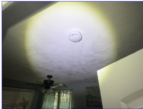
Smoke and CO alarm
