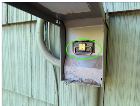
Electric service disconnect
