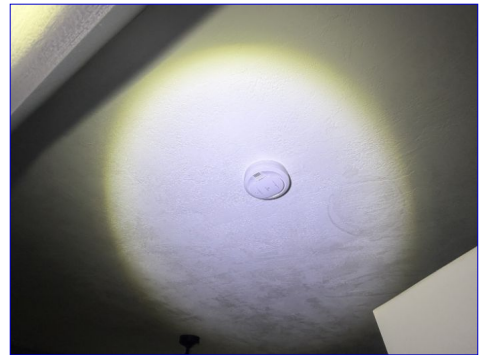
Smoke and CO alarm
