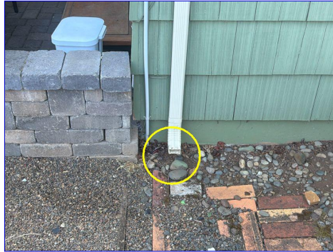
Downspout discharges near foundation
