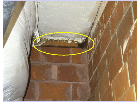
Hole in fire separation wall
