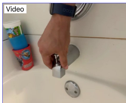
Loose tub faucet
