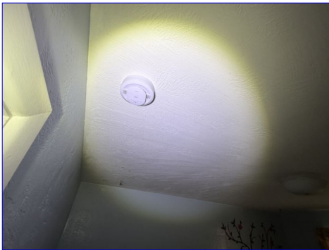
Smoke and CO alarm
