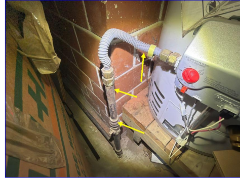
Missing sediment trap
