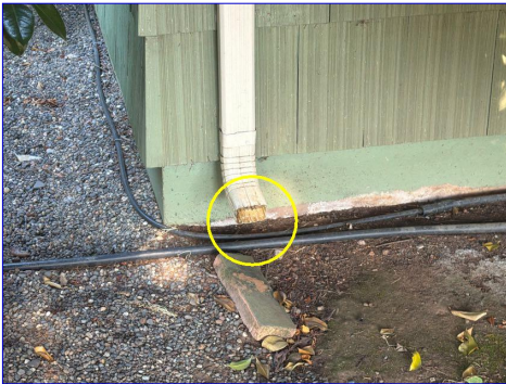
Downspout discharges near foundation
