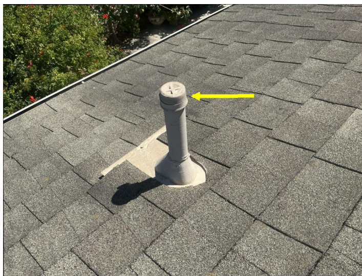
The plumbing vent over the laundry room has been capped. We recommend a qualified plumbing contractor evaluate this and service or correct as needed.
