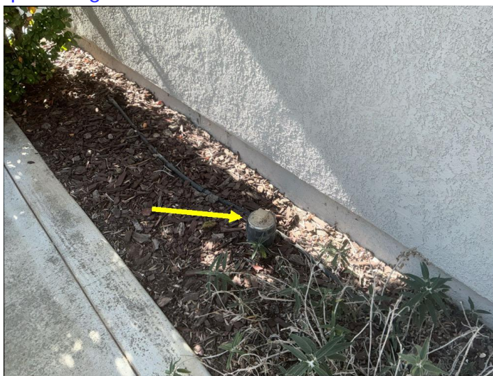
A clean-out is located at the rear.
