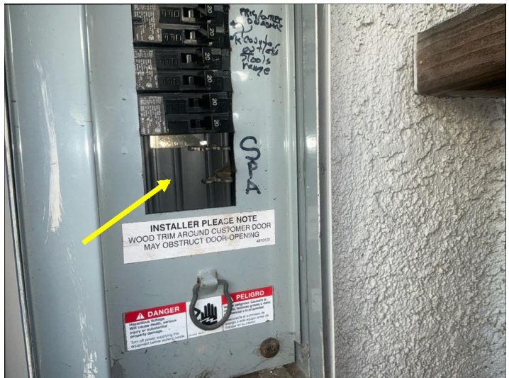
There are voids or open knockouts in the interior cover of the main electrical panel that should be covered.
