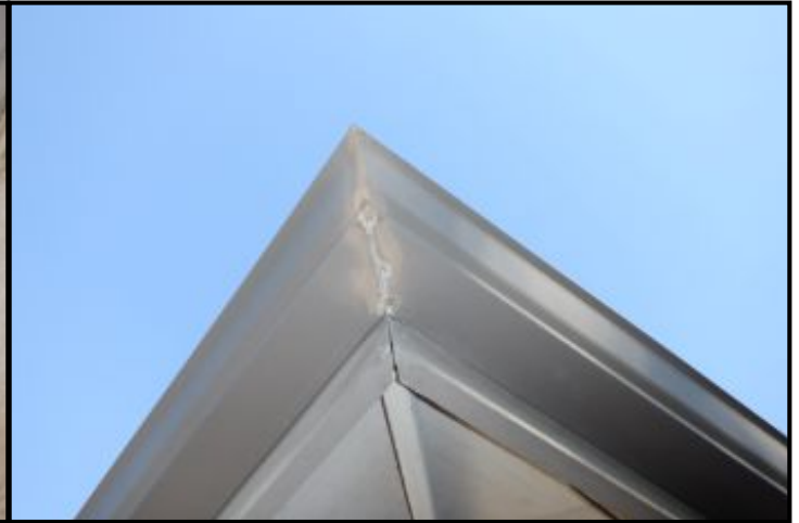
Gutter leaks noted
