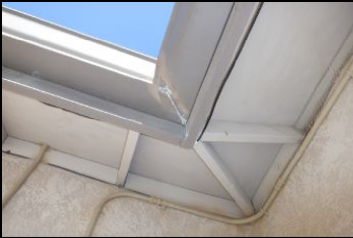
Gutter leaks noted
