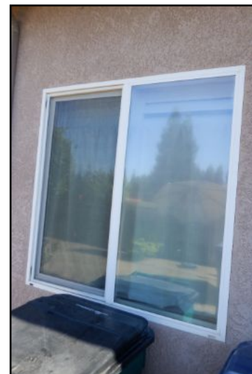
Primary bathroom window is fogged & UV discoloration
