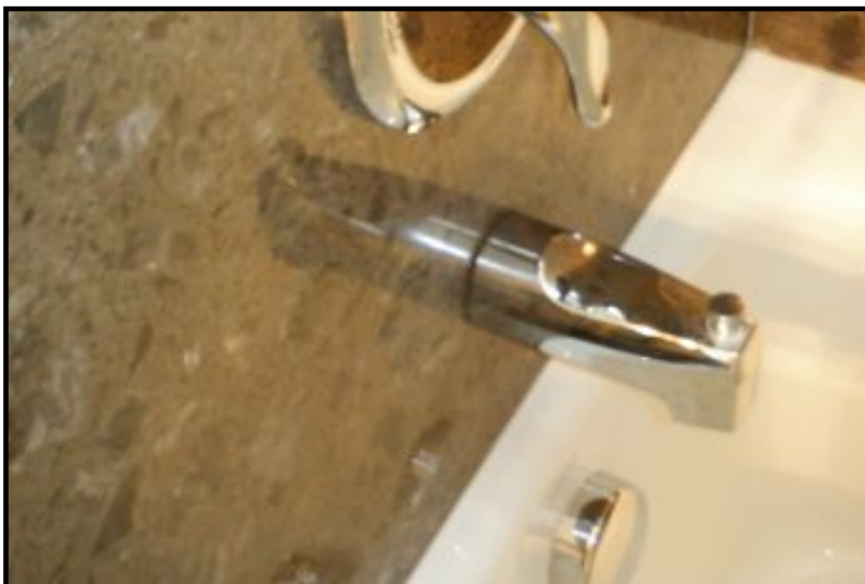
Caulking needed at bathtub spout to wall
