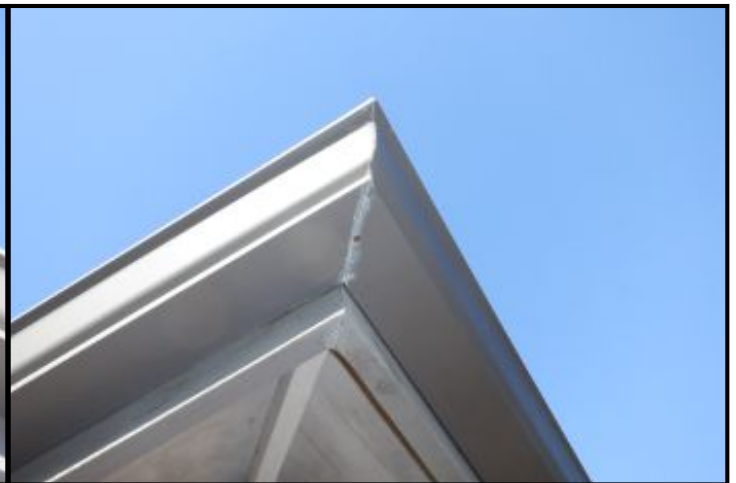
Gutter leaks noted
