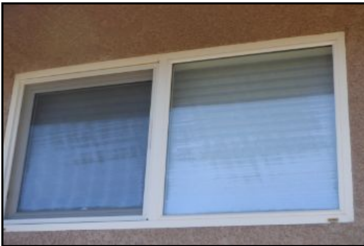
UV discoloration noted at window
