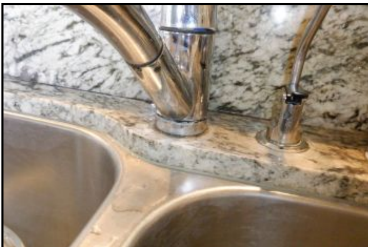
Kitchen sink faucet was leaking
