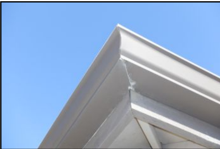
Gutter leaks noted
