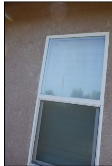
UV discoloration noted at window
