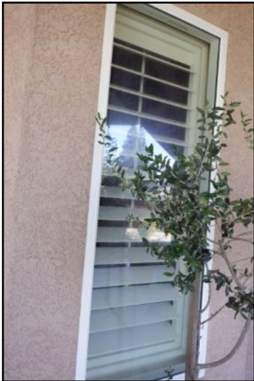
UV discoloration noted at window
