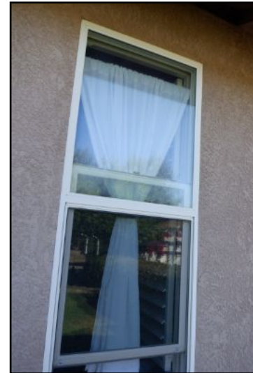
UV discoloration noted at window
