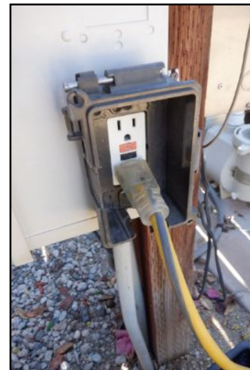
Pool GFCI outlet does not trip off
