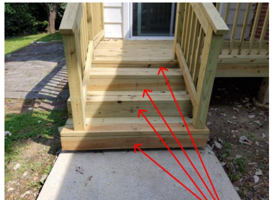
Photo 13: Deck Trip Hazard at Steps.
