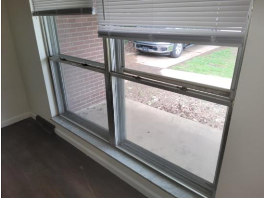
Photo 25: Old Windows - Mild Disrepair.
