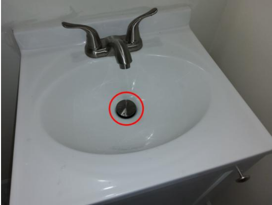
Photo 23: Drain Stopper Inoperative.
