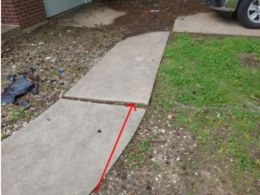
Photo 10: Walkway Trip Hazard.
