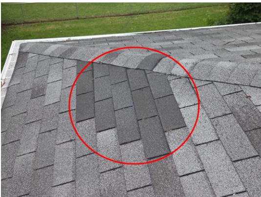
Photo 7: Prior Repairs Noted.
