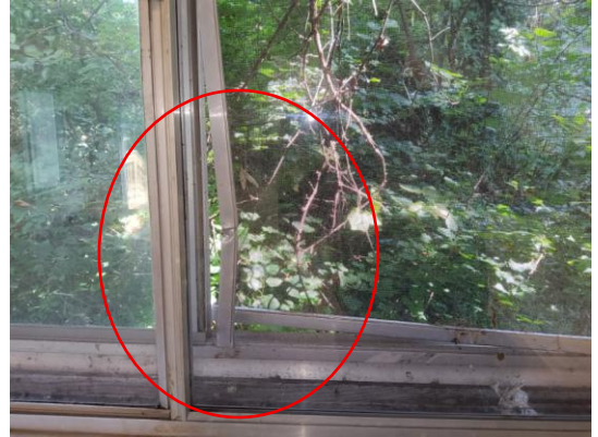
Photo 26: Old Windows - Mild Disrepair.
