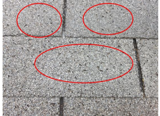
Photo 4: Roofing Nearing End of Life Cycle.
