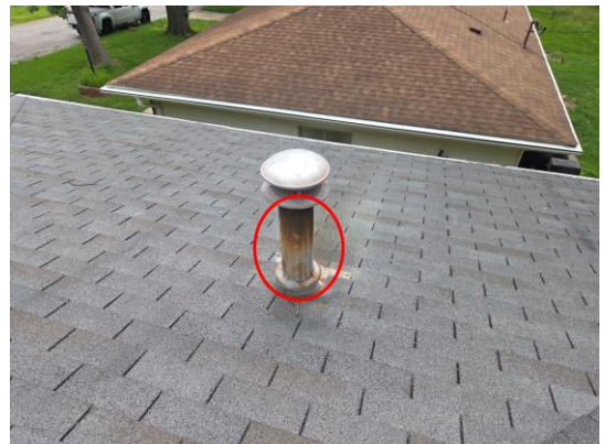
Photo 8: Surface Rust, Paint.
