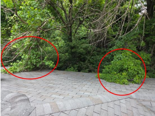
Photo 3: Tree Trimming Needed.
