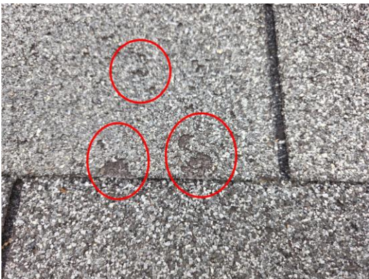
Photo 5: Roofing Nearing End of Life Cycle.
