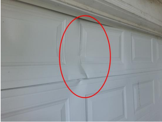
Photo 16: Overhead Door Minor Damage.
