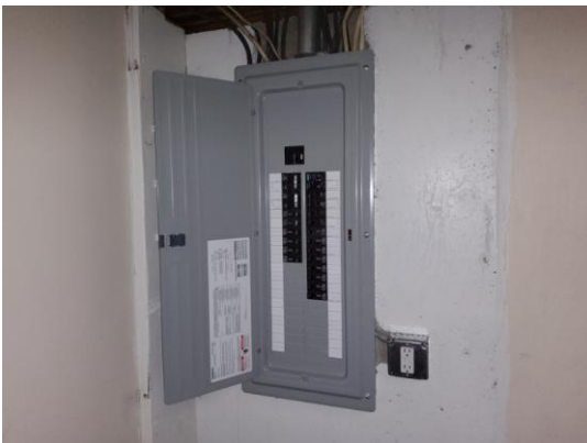
Photo 19: No Inspection Sticker.
