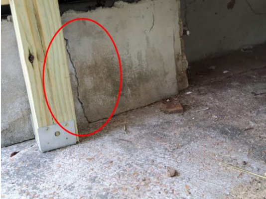
Photo 1: Cracks Moderate - Settling.
