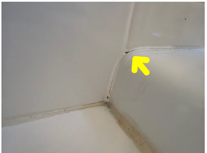
One or more open seams in the tub area need to be caulked or re-grouted to forestall moisture intrusion.
