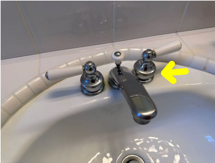
The sink faucet leaks around the stem and should be repaired.
