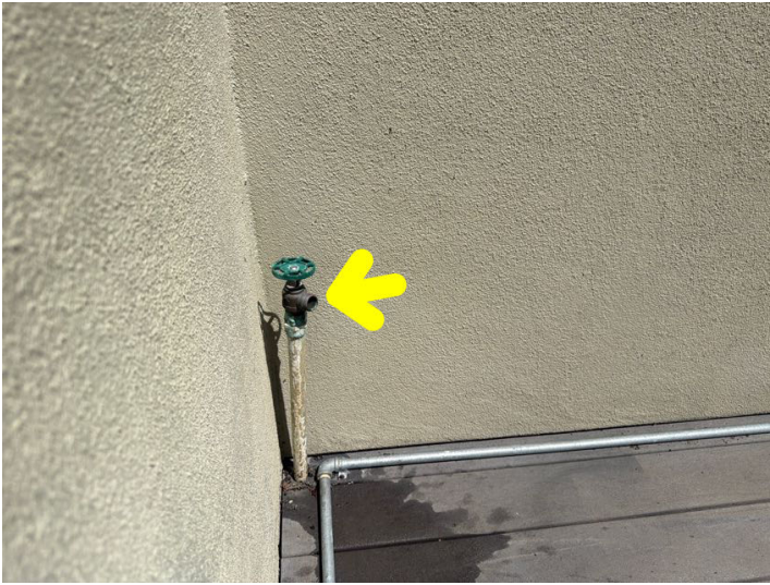
A hose bib at the rear is leaking and should be evaluated and serviced by a qualified plumbing contractor.
