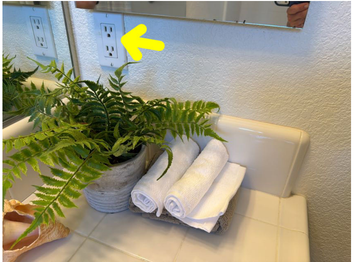
One or more bathroom sink outlets have an open-ground, and should be evaluated and serviced by a licensed electrical contractor.
