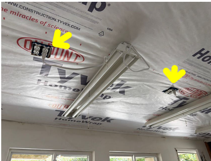
One or more outlet covers are missing and should be installed.
