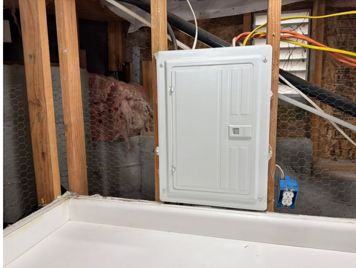
The sub panel is located in the crawlspace.
