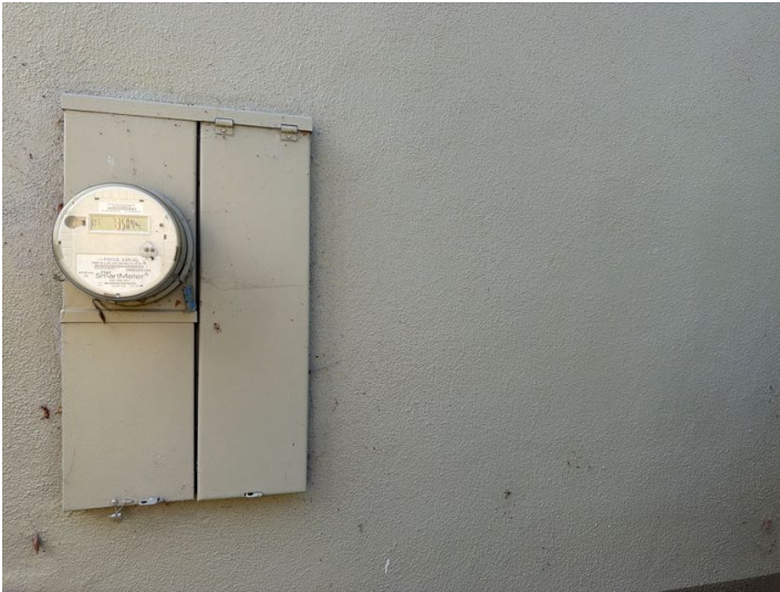
The residence is served by a 100 amp main electrical panel, located at the left side of the home or unit.
