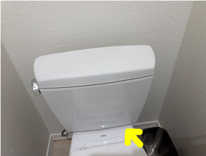
The toilet tank is loose, and should be secured, as this could be a safety hazard.
