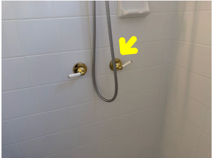
The shower faucet leaks around the stem while in use, and should be repaired.
