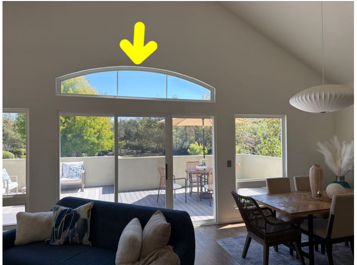
One or more windows may have a broken hermetic seal, which you may wish to have replaced. This is evident from fogging or condensation forming between the panes of glass, which implies that the seal has failed.
