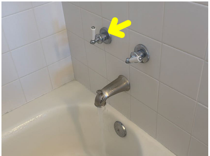
The shower valve handle is loose or does not function properly and should be serviced.
