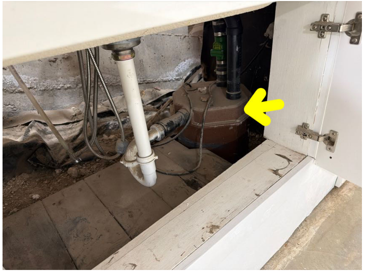
The waste and drainage system includes a sewage ejector system that we do not have the expertise to evaluate. Because part of the living space is located lower than the public street, a sewage ejector is used to pump waste to the street. You should ask the sellers about its operation and when it was last serviced.
