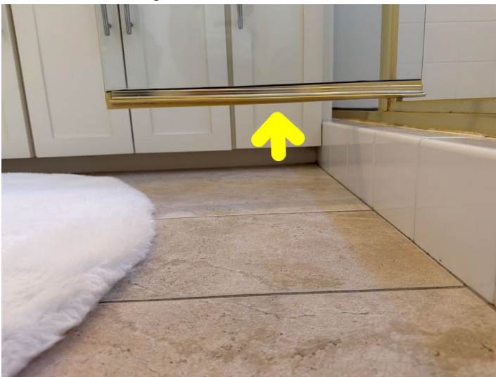
The shower door seal is missing or damaged, and should be serviced.
