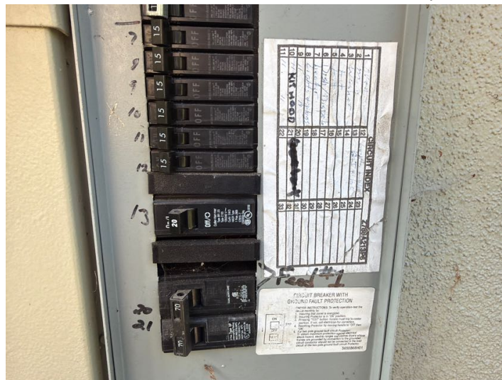
Various circuits within the main electrical panel are not labeled, and this condition should be serviced by a qualified electrical contractor so that the appropriate load calculations and breaker sizes can be determined.
