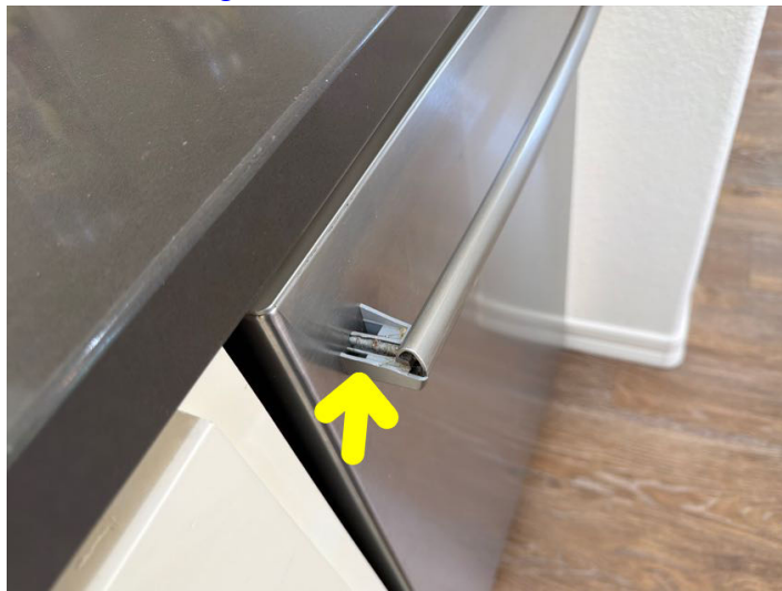
The door handle is loose or damaged and should be secured.
