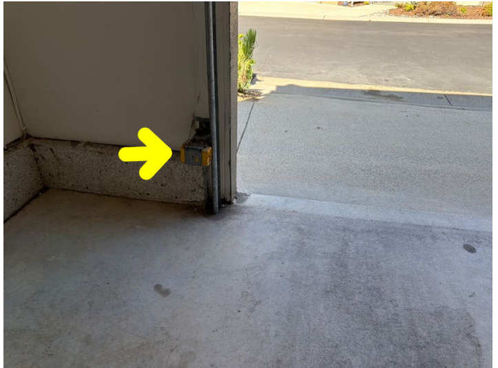
The infrared auto-reversing sensor mechanisms are functional but located higher than the recommended six inches above grade.
