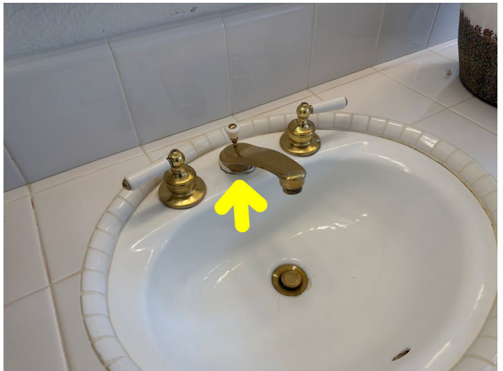
The left sink faucet is loose, and should be secured.
