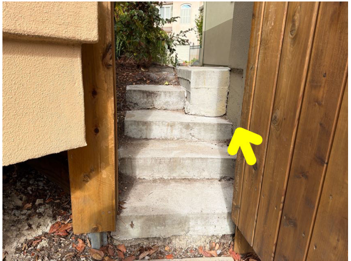
Current building standards require handrails to be installed on steps which have 4 or more risers, which is particularly important if children or the elderly visit or occupy this property.
