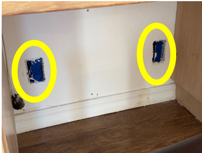
One or more outlet covers are missing and should be installed.
