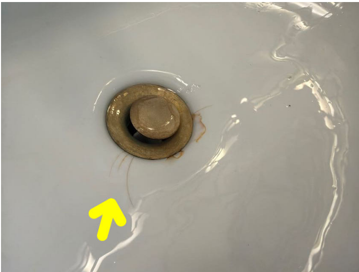
The bathroom sink is cracked but not leaking, but will obviously be susceptible to leaks.
