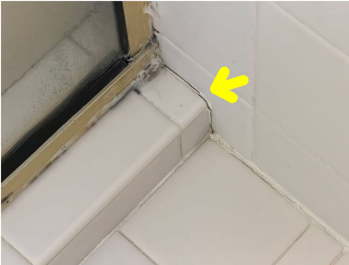
One or more open seams in the shower area need to be caulked or re-grouted to forestall moisture intrusion.
