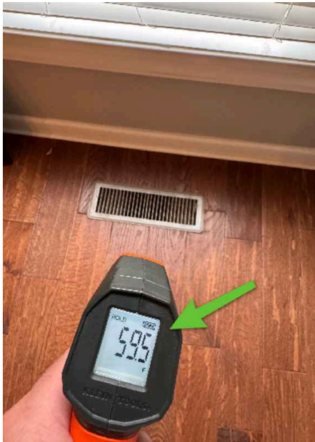
First floor supply temperature
