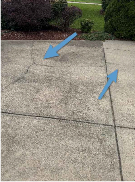
Typical slab cracks noted in driveway
