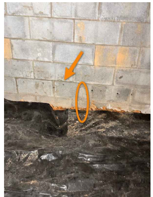
Possible termite tube at front center of the crawlspace. Drill marks for treatment were also noted.
