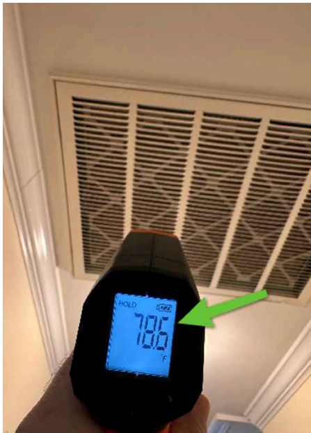
Second floor return temperature
