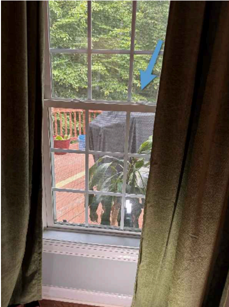
Several windows did not stay open
