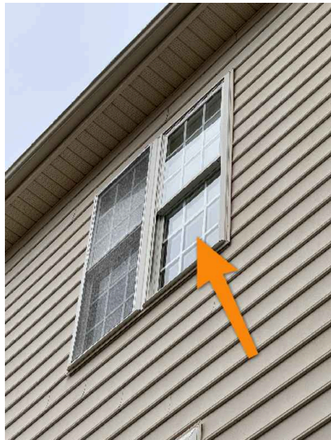
Example of missing Screen
