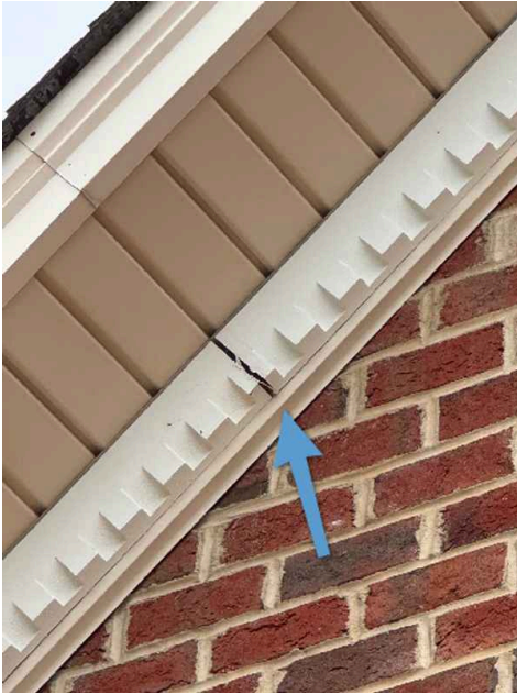
Multiple gaps noted in trim work
