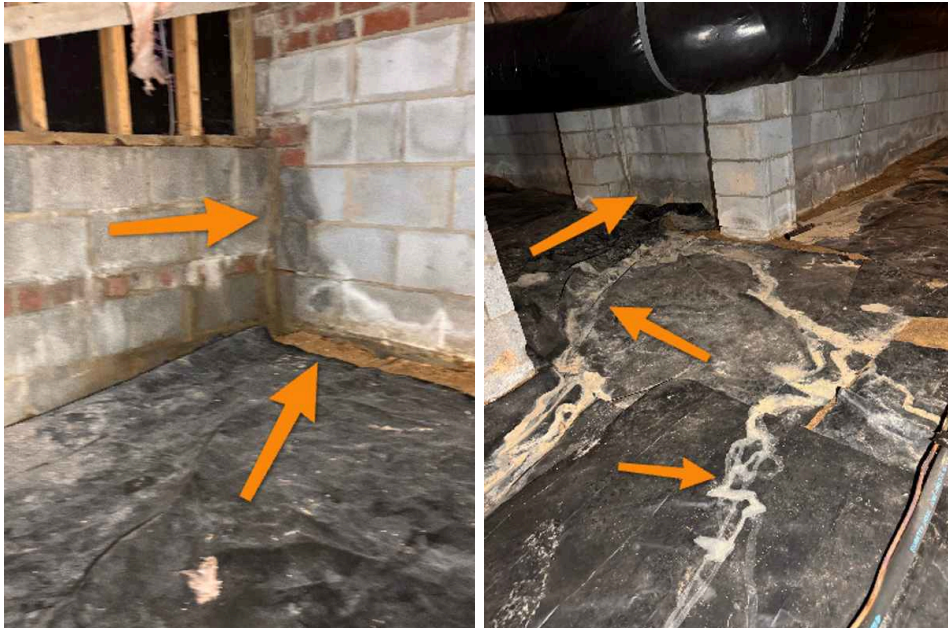
Evidence of water intrusion at the front center of the crawlspace
