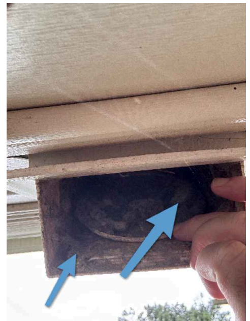
Lint buildup at exterior dryer vent
