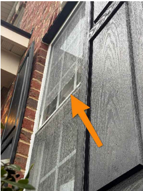
Example of torn screen
