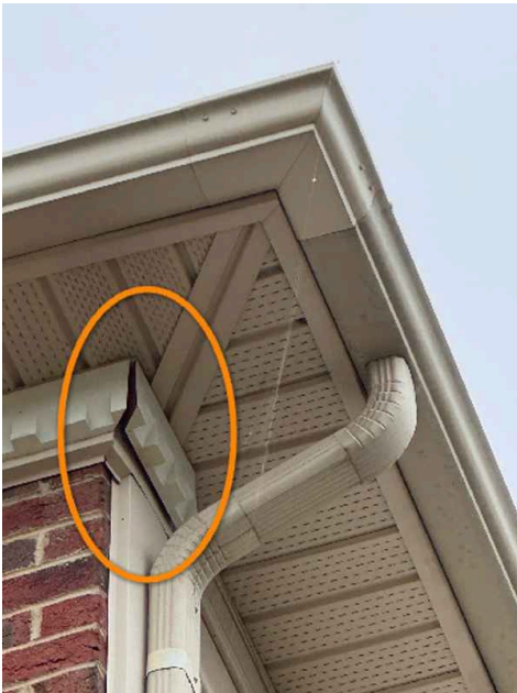
Loose piece at front right corner
