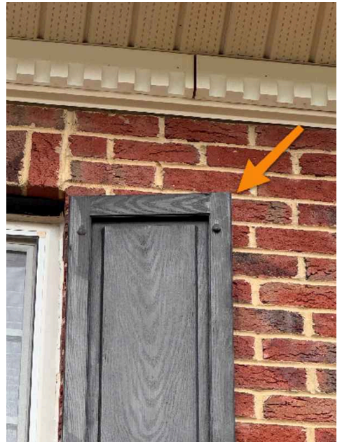
Several shutters appear loose and need securing
