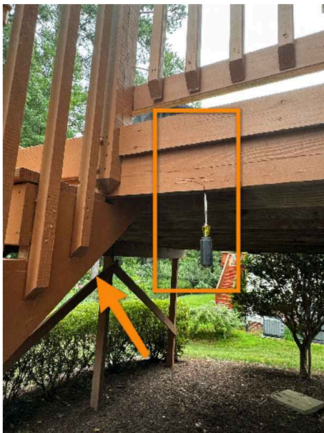
Exterior band member that supports stairs is cracked and needs review
