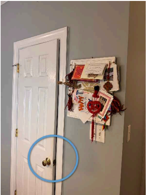
Multiple doors throughout the home do not latch and need adjustment
