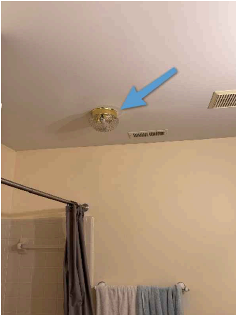
Multiple lights throughout the home did not come on and probably need new bulbs
