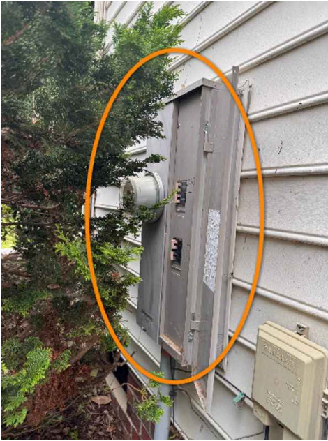
Exterior panel access is blocked by vegetation
