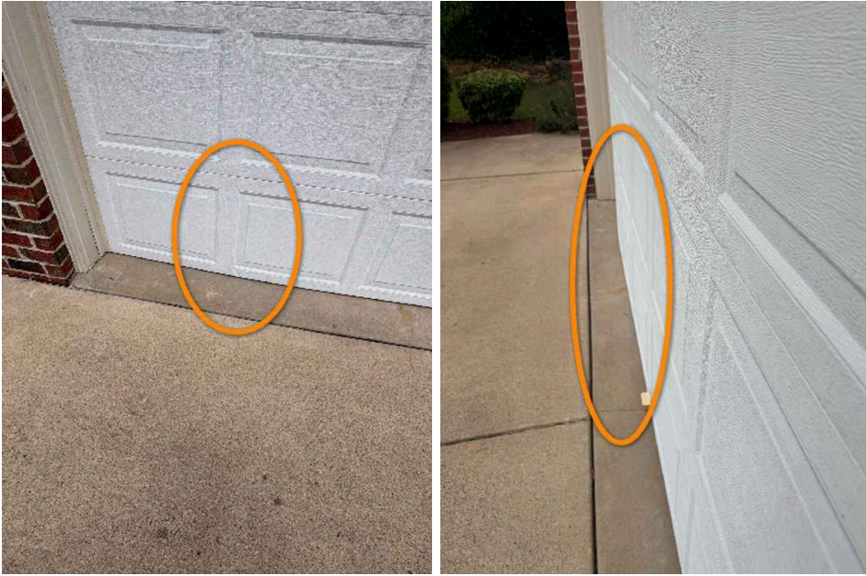
Dented area of bottom panel on left side
