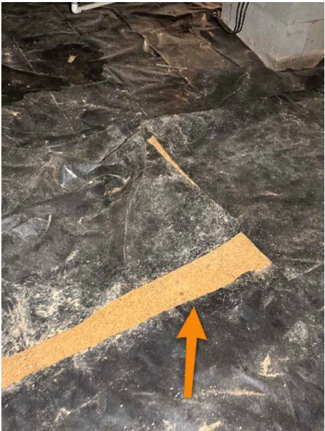
Vapor barrier bunched in multiple spots
