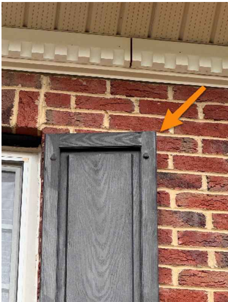
Several shutters appear loose and need securing
