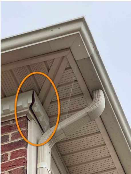
Loose piece at front right corner
