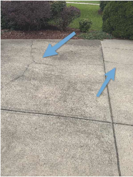
Typical slab cracks noted in driveway
