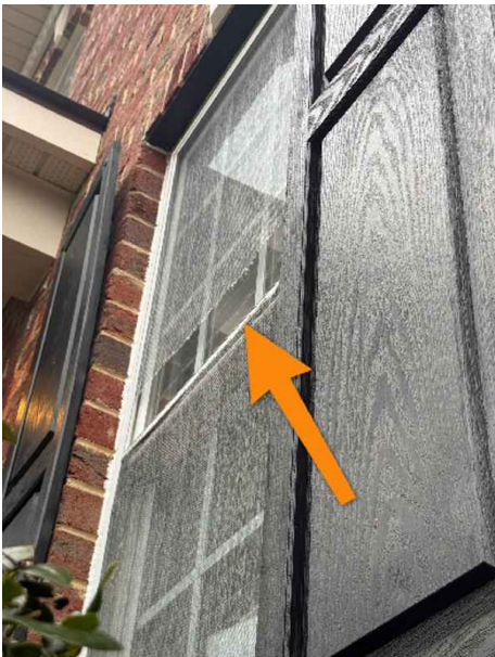
Example of torn screen
