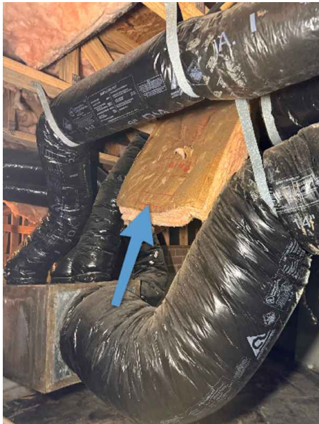
Several pieces of insulation have fallen down in the crawlspace
