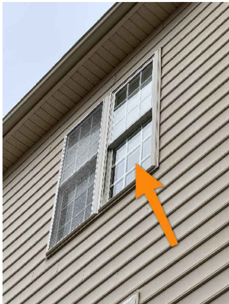
Example of missing Screen
