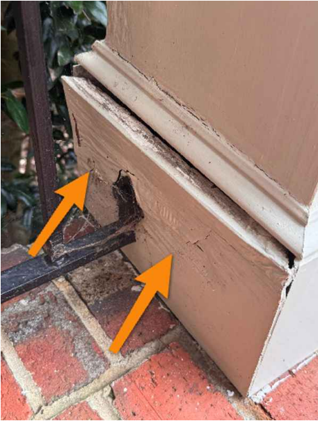
Rot at right front porch post on back side
