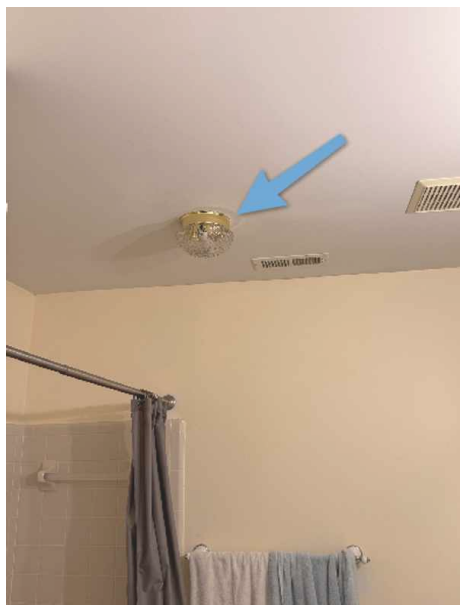
Multiple lights throughout the home did not come on and probably need new bulbs
