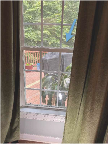
Several windows did not stay open
