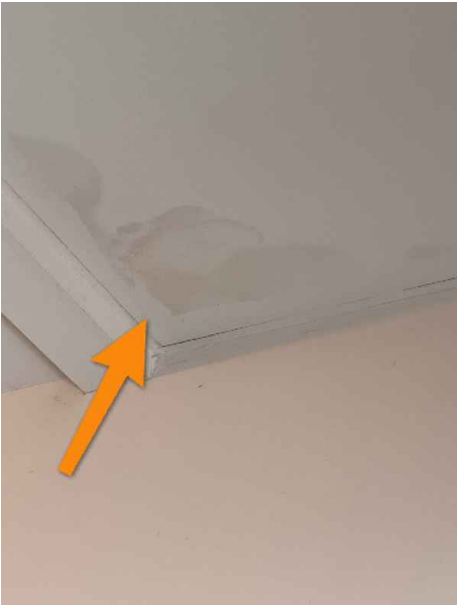
Water stain in garage ceiling at right middle
