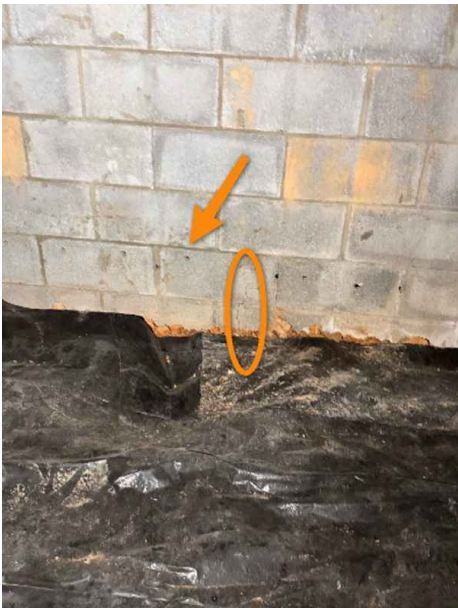
Possible termite tube at front center of the crawlspace. Drill marks for treatment were also noted.
