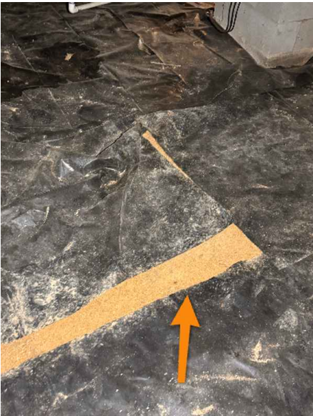
Vapor barrier bunched in multiple spots
