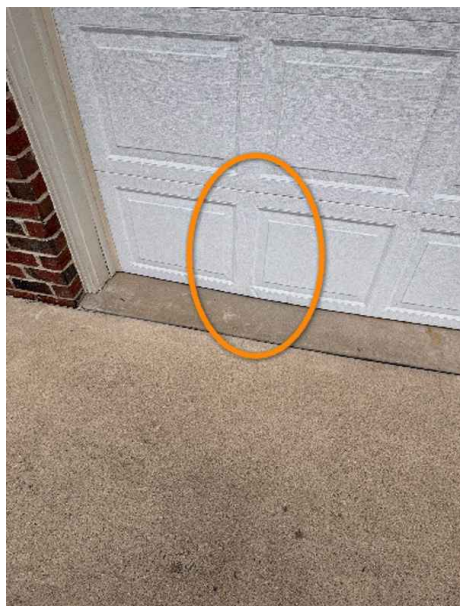
Dented area of bottom panel on left side
