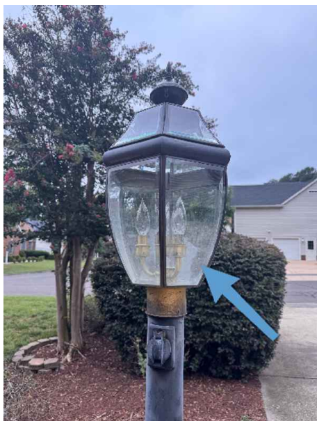
The front yard light did not come on and the cap is very loose
