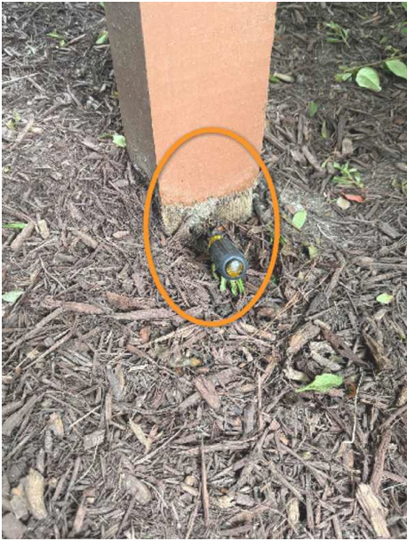
Several deck posts have significant deterioration at grade level
