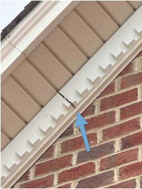
Multiple gaps noted in trim work
