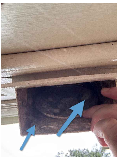
Lint buildup at exterior dryer vent
