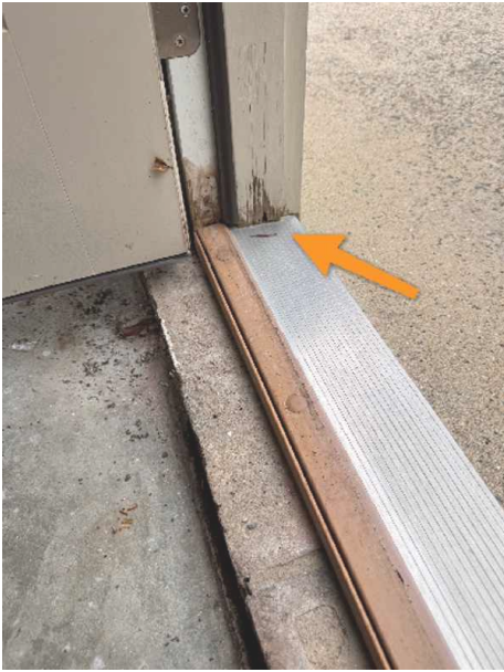
Exterior doors and trim had noticeable amounts of rot along bottom
