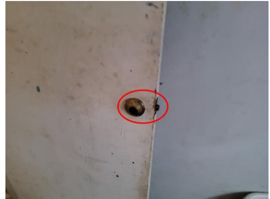
Photo 34: Door Hardware Missing.
