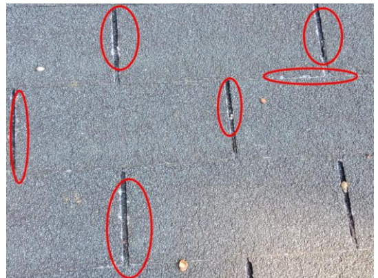
Photo 6: Roofing Nearing End of Life Cycle.
