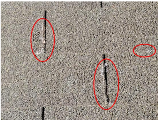
Photo 5: Roofing Nearing End of Life Cycle.
