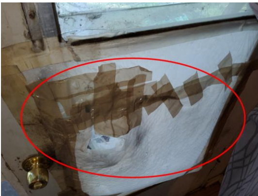
Photo 35: Door Physical Damage.
