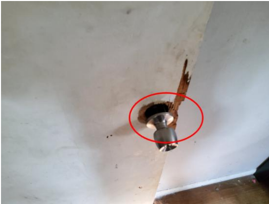
Photo 33: Door Hardware Missing.
