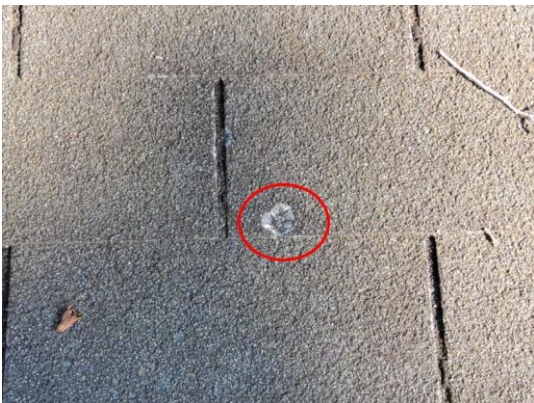
Photo 7: Roofing Nearing End of Life Cycle.
