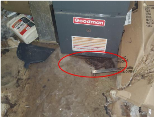
Photo 26: Active Condensate Leakage.
