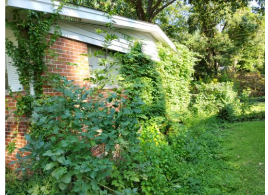
Photo 11: Vegetation on Exterior Walls.
