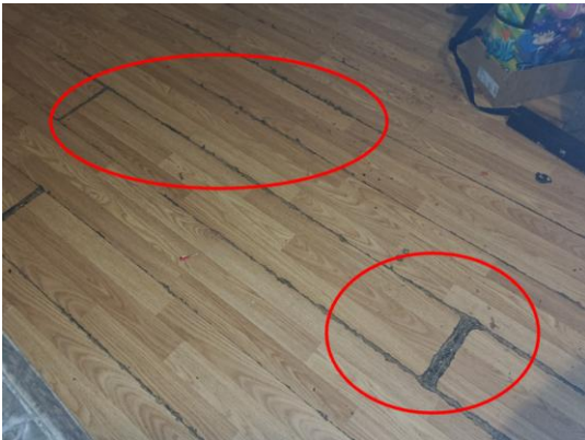
Photo 47: Laminate Floor Water Damage.
