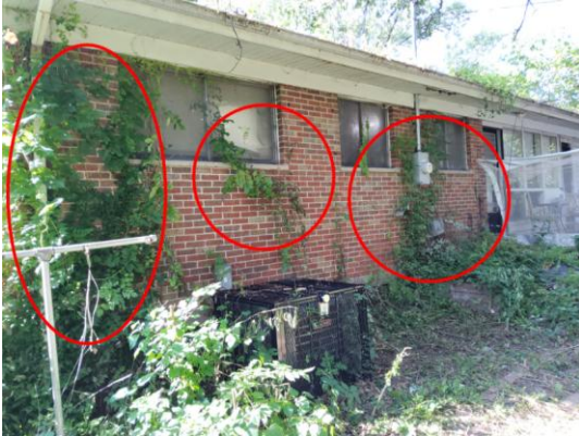
Photo 10: Vegetation on Exterior Walls.
