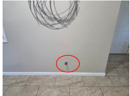
Photo 15: Ungrounded 3-prong Outlet.
