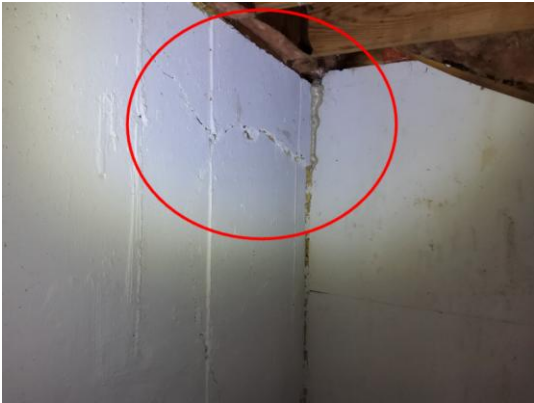
Photo 1: Cracks Moderate - Bowing.
