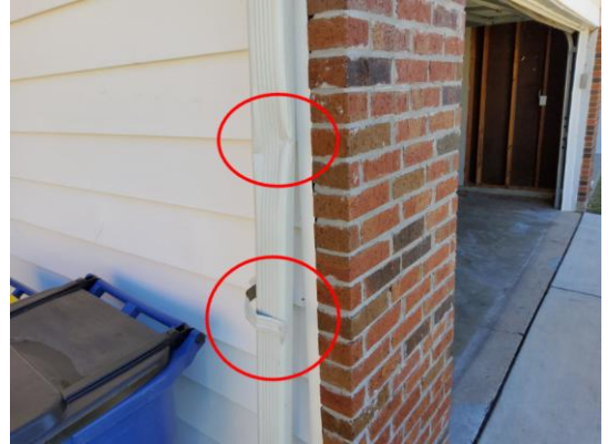
Photo 5: Downspout Loose / Damaged.
