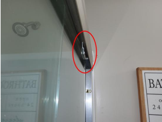
Photo 19: Shower Door Rollers Poor.
