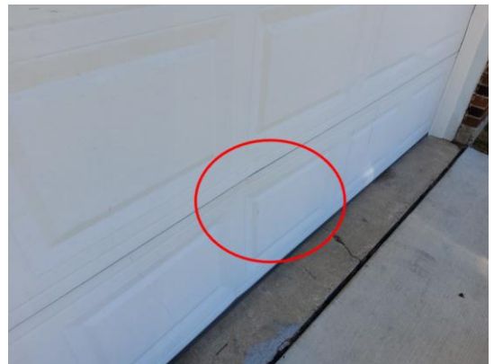
Photo 10: Overhead Door Minor Damage.
