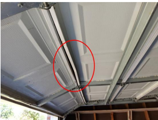
Photo 11: Overhead Door Minor Damage.
