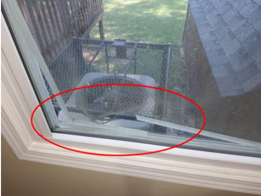
Photo 22: Window Screen Damaged.
