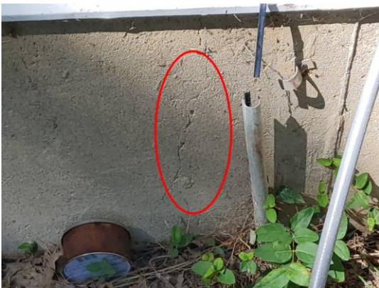
Photo 3: Cracks Minor - Settling.
