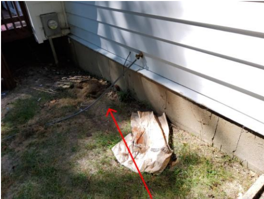
Photo 7: Grading Improvement Needed.
