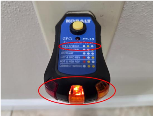
Photo 14: Ungrounded 3-prong Outlet.
