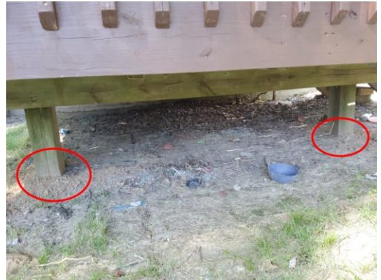
Photo 8: Wood-Soil Contact of Deck Post.
