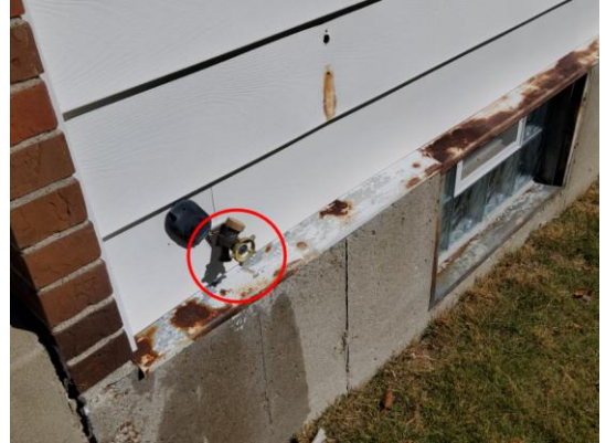
Photo 20: Hose Bib Loose .
