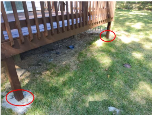
Photo 9: Deck Posts Mounted Directly in Concrete .
