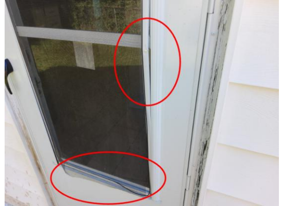
Photo 23: Window Screen Damaged.
