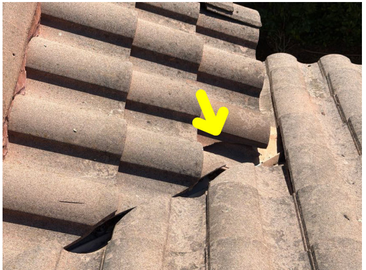
There are one or more cracked or broken tiles that should be serviced by a licensed roofing contractor.
