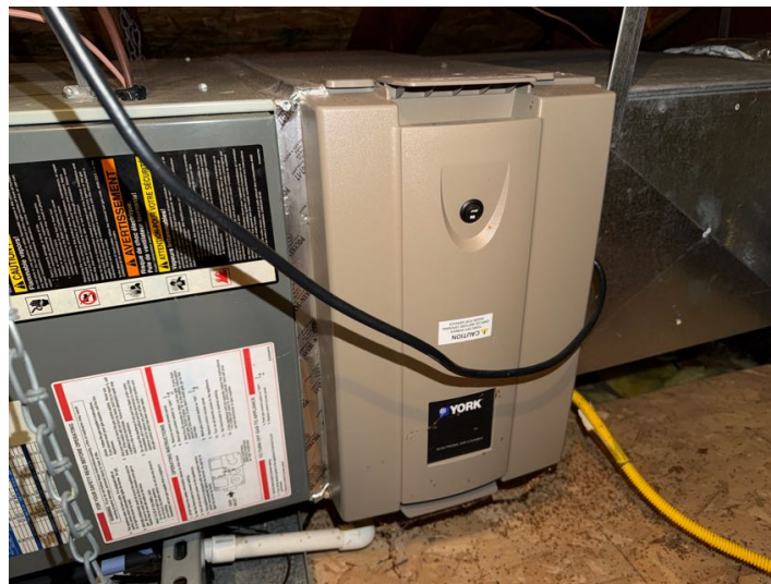
The furnace filter is a specialized unit that should be explained and demonstrated by the seller or the HVAC company that performed the installation. You may also refer to the operation manual that was supplied with the unit.
