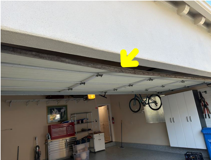
The garage door has cosmetic damage that you should view for yourself.
