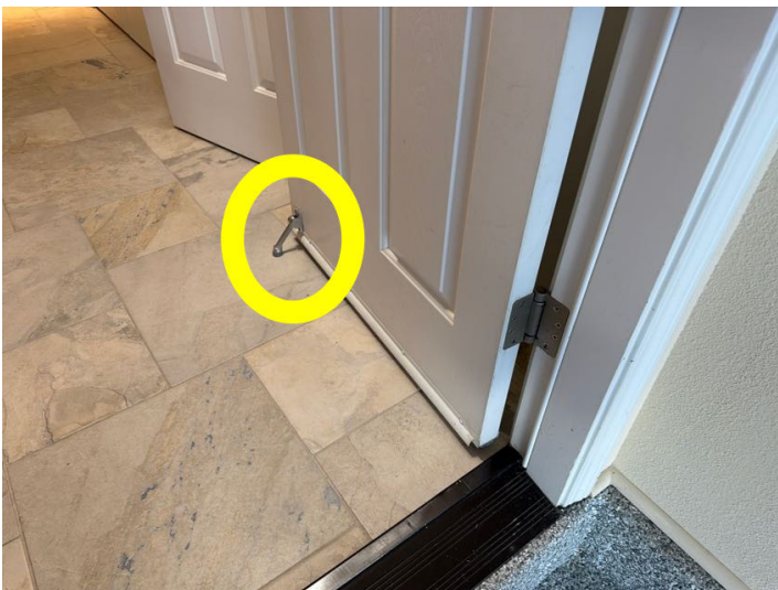
The fire rating of the house entry door has been nullified by the addition of a foot operated door stop, and you may wish to have the door stop removed for optimal safety.
