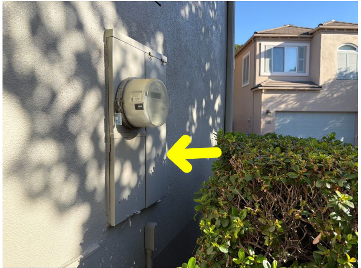
The main panel does not have thirty-six inches of clear space in front of it to facilitate an emergency disconnect, a condition which should be corrected.
